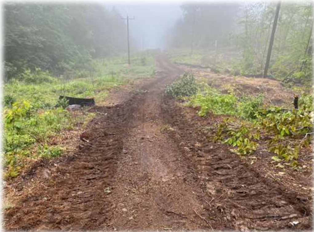
Photo #2: Water bars have been created along the corridor access road. The bars flow to a stabilized area with silt fence barrier to collect potential sediment wash. CLT forwarder has crushed the bar and will recreate the bar as they work themselves out later in the day. Disturbed areas of the road and structure equipment install pads are hay mulched.
