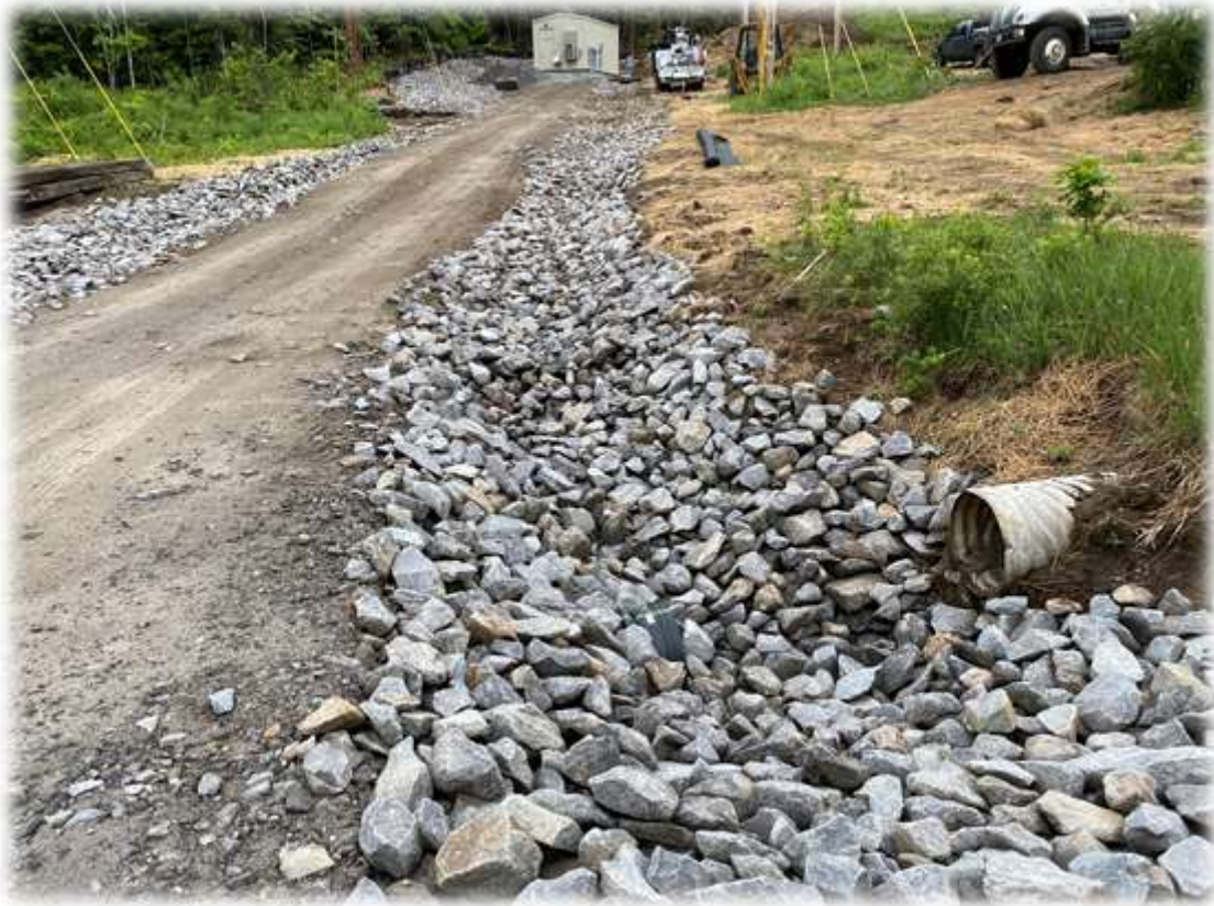
Photo #7: The remaining short section of the SCADA driveway ditch has been constructed with riprap on fabric.
