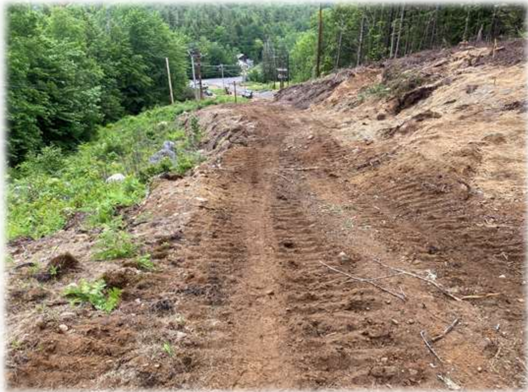
Photo #6: This area remains stable, but the water bars installed do not have any stabilized outlets. Sediments that are diverted by the bar will flow into vegetated areas and need to be removed.
