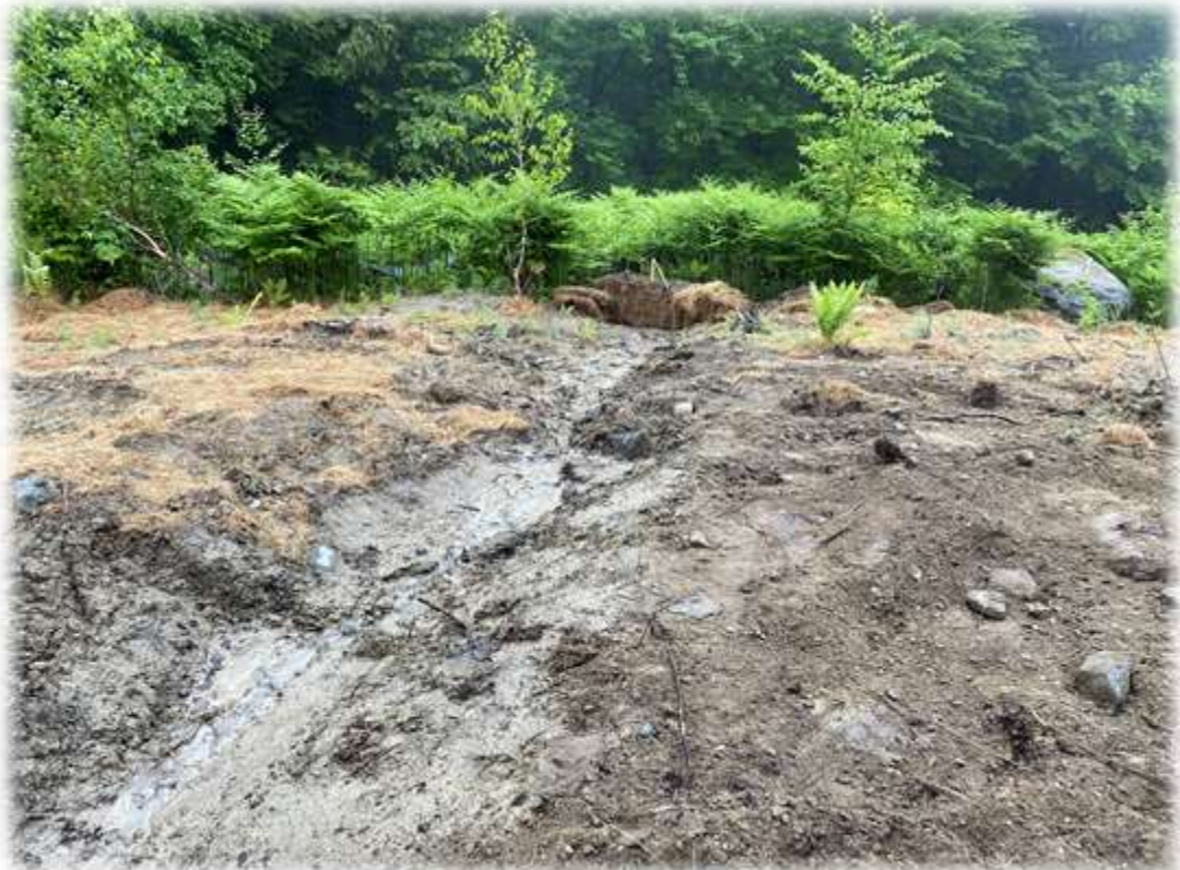
Photo #4: The Contractor has removed sediment from the water diversion bar and stabilized outlet near P-19
