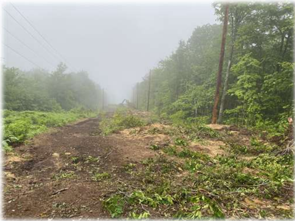
Photo #1: The upper portion of the transmission corridor access road coming into the RoxWind Towers portion of the project has been constructed and structures set. CLT is back onsite to cull the safety "danger" trees from the corridor using hand labor and a forwarder.
