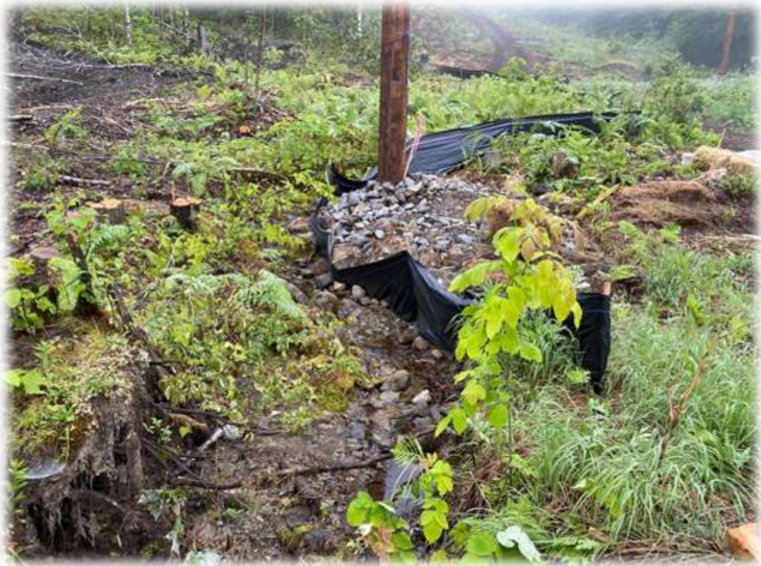
Photo #3: Structure P-23 has been placed along the side of a stream. Silt fence and rock have been placed to minimize impact to the stream. Some of the rock that has fallen into the stream has been removed. The downslope staked hay bales within the stream have also been removed.
