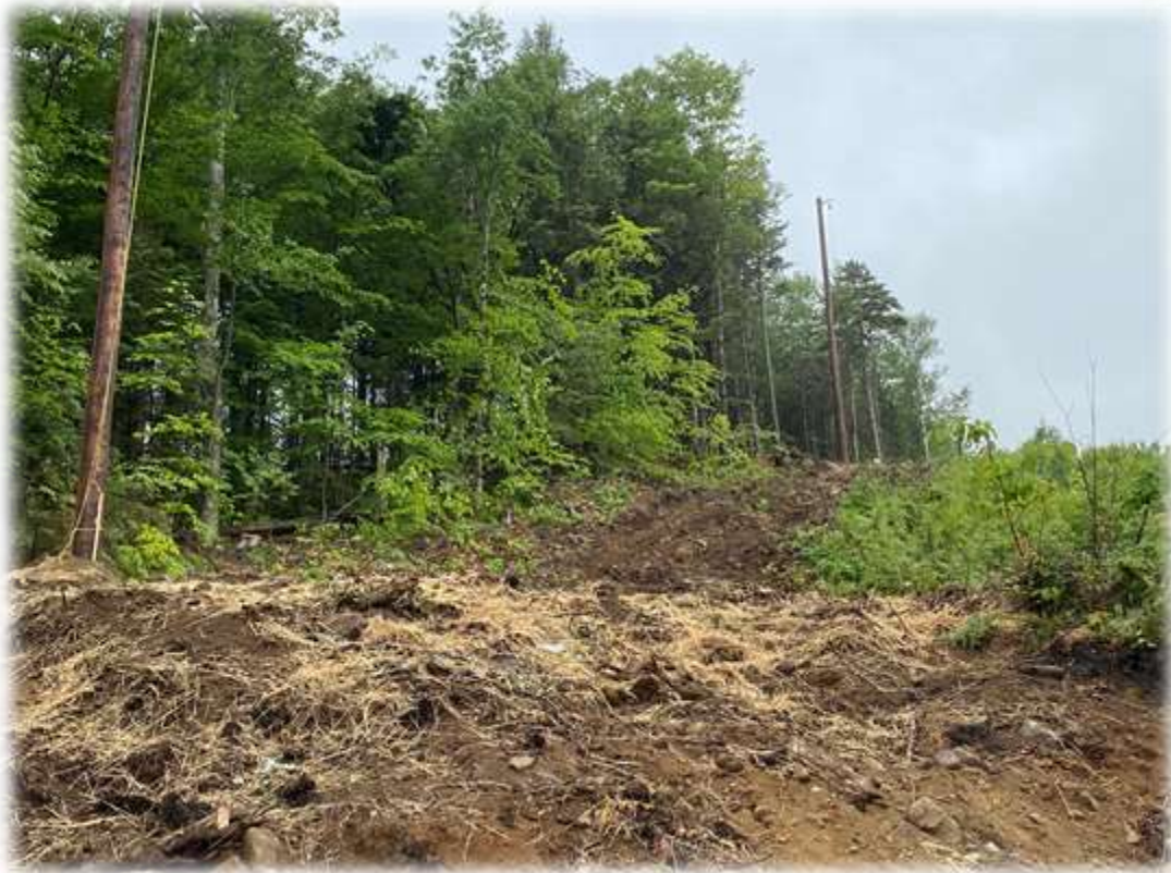
Photo #5: CLT has disturbed a new area adjacent to the woods line that needs hay mulch (work in progress).
