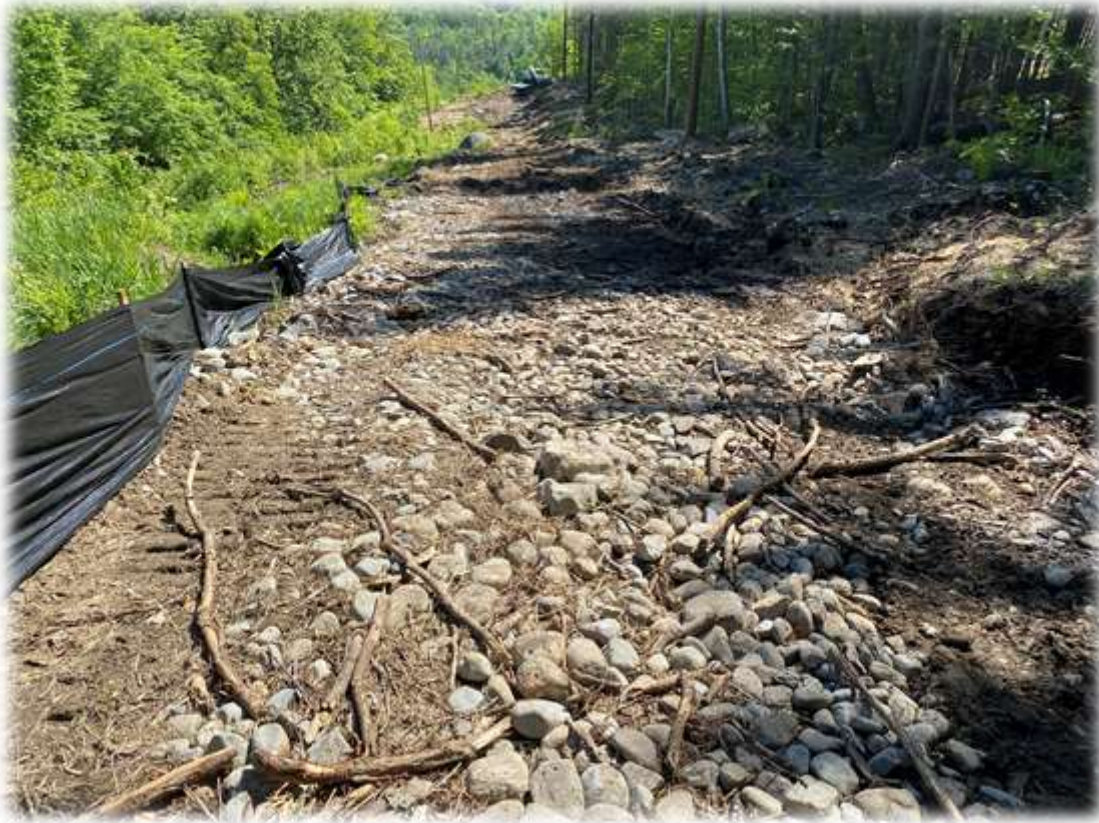
Photo #5: Stone has been added to the access road. It will need to be removed during restoration.
