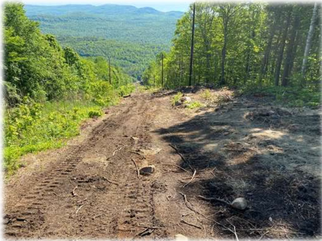
Photo #2: Water bars have been created along the corridor access road. The bars flow to a stabilized area with silt fence barrier to collect potential sediment wash. Disturbed areas of the road and structure equipment install pads are hay mulched.
