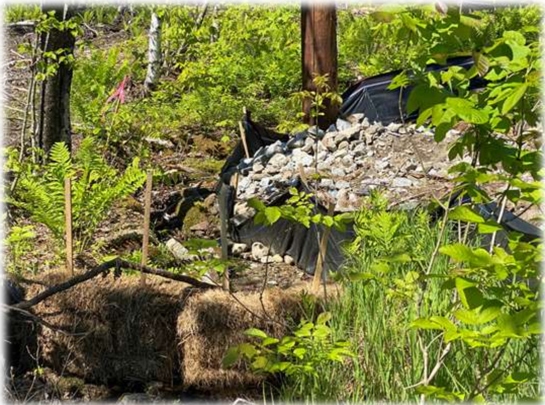
Photo #4: Structure P-23 has been placed along the side of a stream. Silt fence and rock have been placed to minimize impact to the stream. The rock that has fallen into the stream needs to be removed. The staked hay bales within the stream need to be removed.
