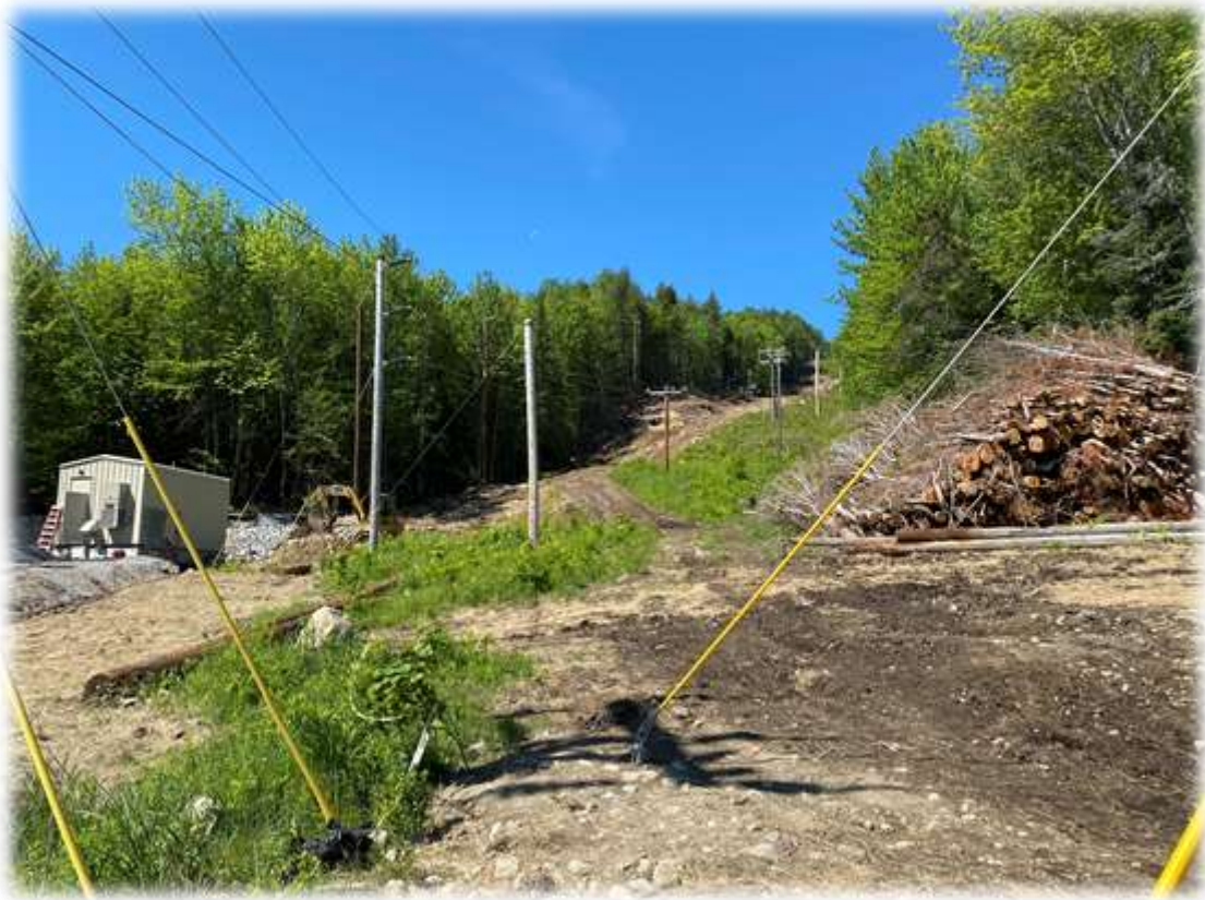
Photo #9: An overview of the lower access road near the SCADA building
