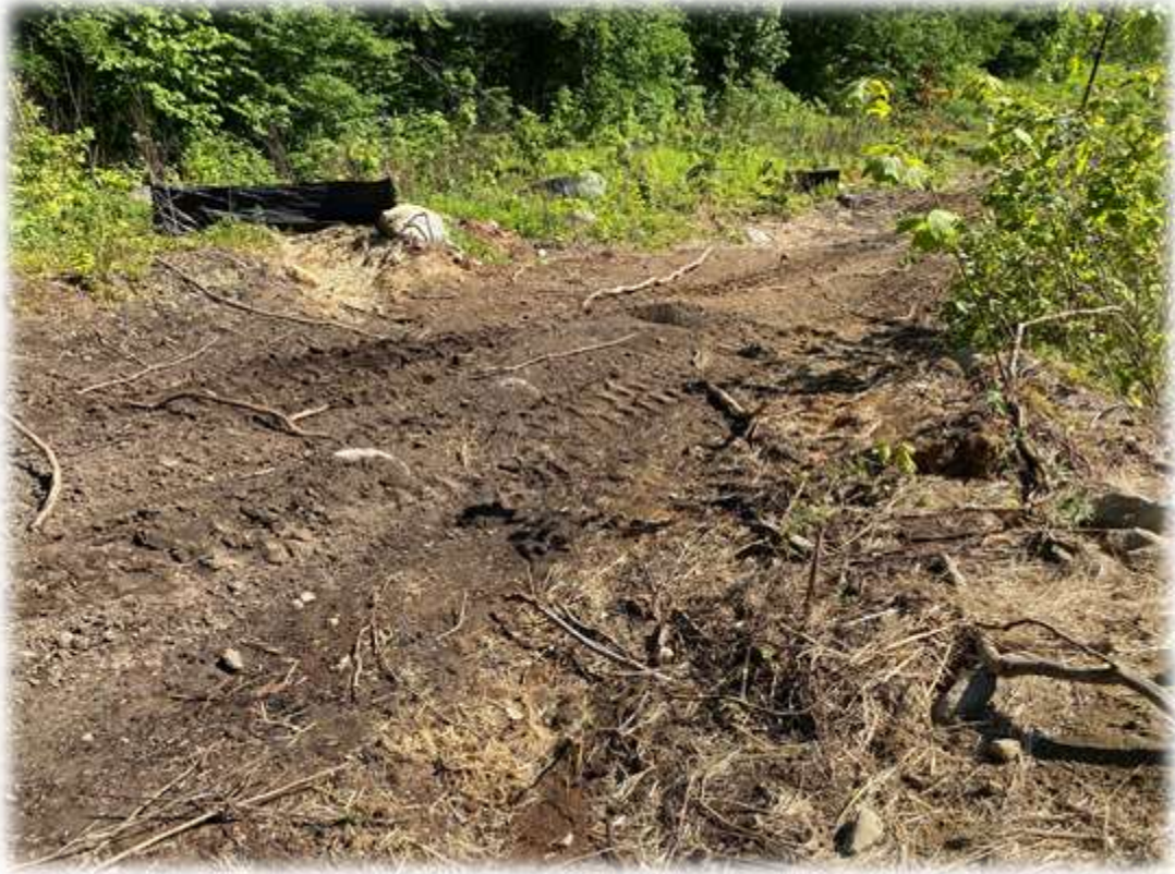
Photo #3: Another example of water bars installed along the corridor access road. The Contractor needs to insure the bars are adequately constructed at the end of each day.
