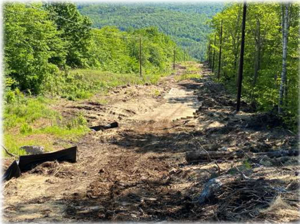
Photo #1: The upper portion of the transmission corridor access road coming into the RoxWind Towers portion of the project has been constructed and structures set. Mats have been installed over a stream and wetland areas.
