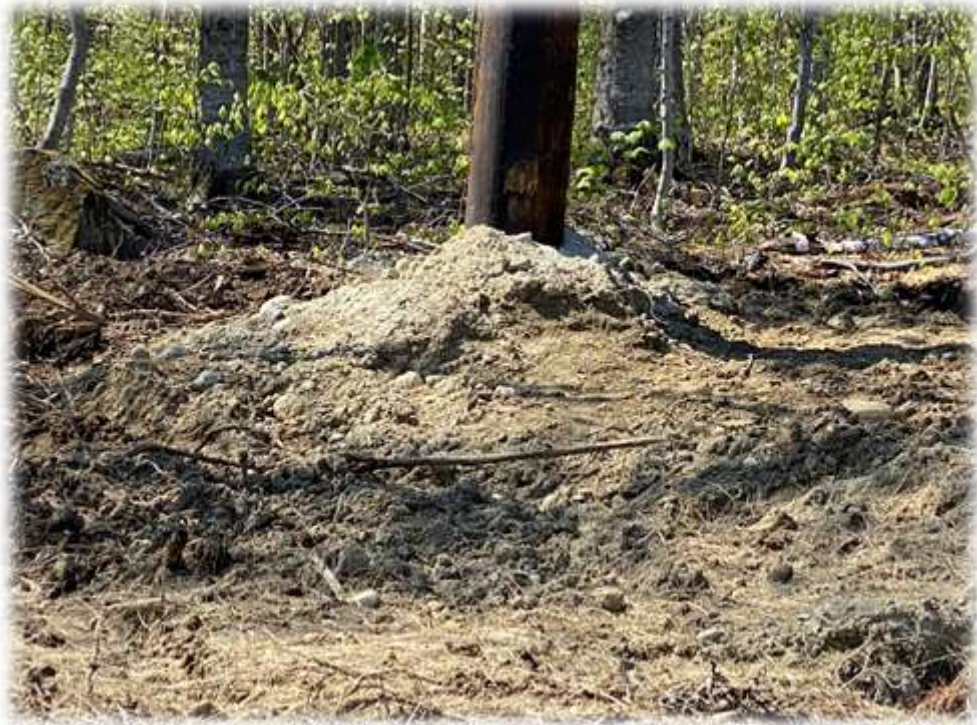
Photo #10: Mulch should be applied to all disturbed soils including pole placement soil haunches.
