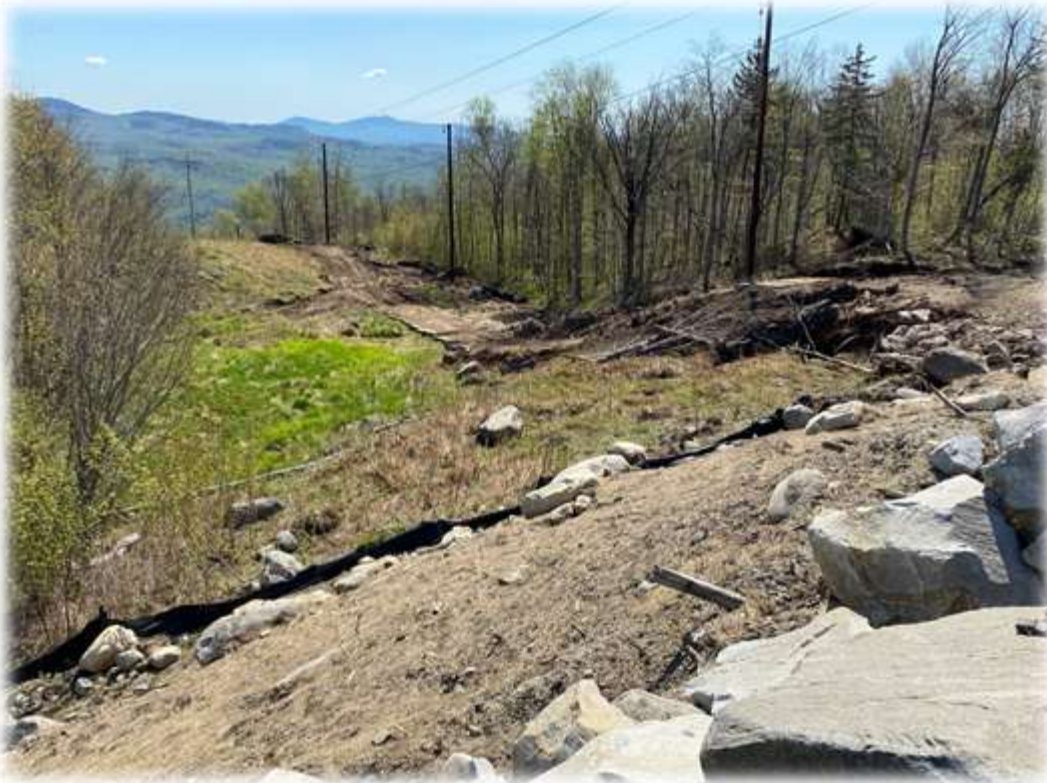
Photo #4: The upper portion of the transmission corridor access road coming into the RoxWind Towers portion of the project has been constructed and structures set. Mats have been installed in wetland areas. A stream is shown on the plans flowing through the matted area. Mats need to be reinstalled to allow unimpeded stream flows.
