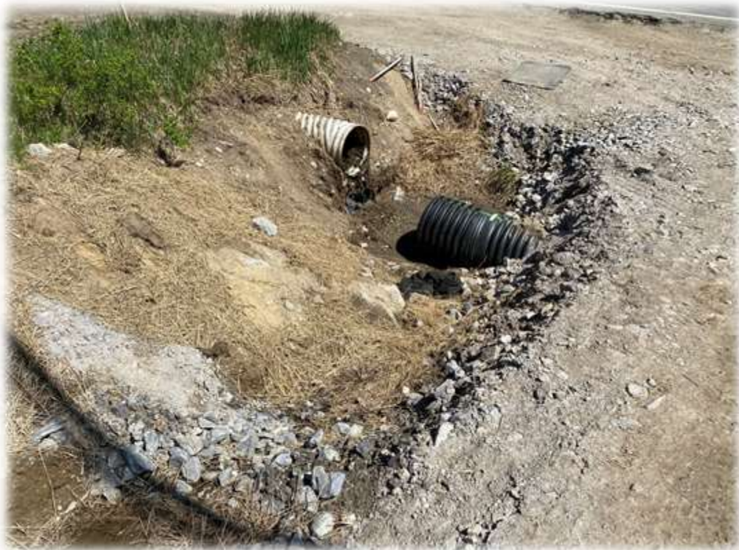
Photo #2: Riprap on fabric protection needs to be installed at the inlet/outlet to the driveway culvert at the entrance to Roxbury Road.
