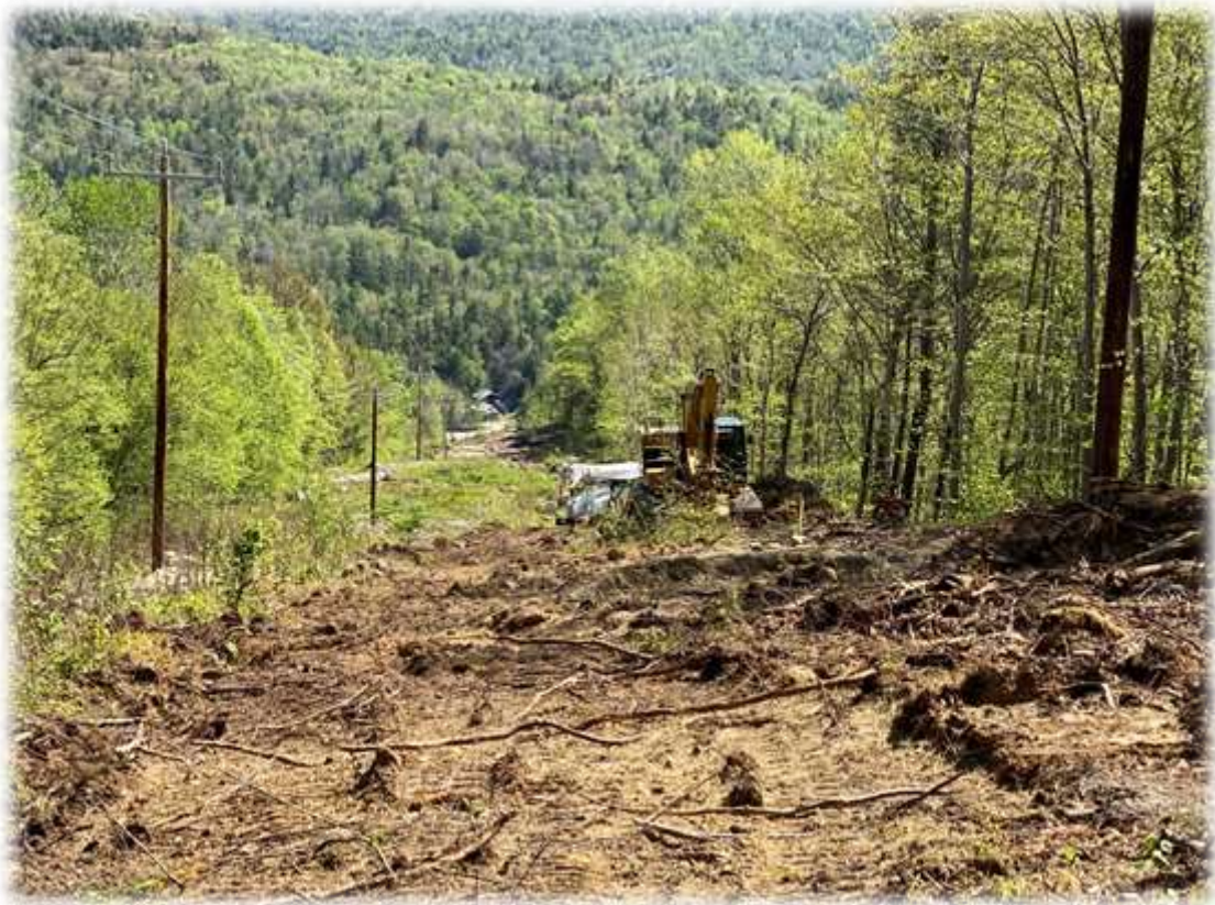
Photo #8: Crews have created access road and installed structures just past existing Section 52 pole 10. Disturbed areas should have hay mulch applied. Access road should have water bars with stabilized outlets.
