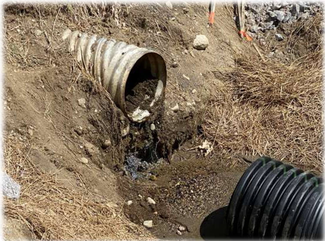
Photo #4: Riprap on fabric protection needs to be installed at the inlet/outlet to the driveway culvert at the entrance to Roxbury Road.
