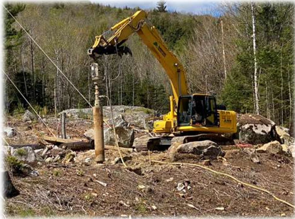
Photo #9: Structure 137-3 "on hold" for construction as the structure was located in the center of a drainage swale with significant flowing water.
