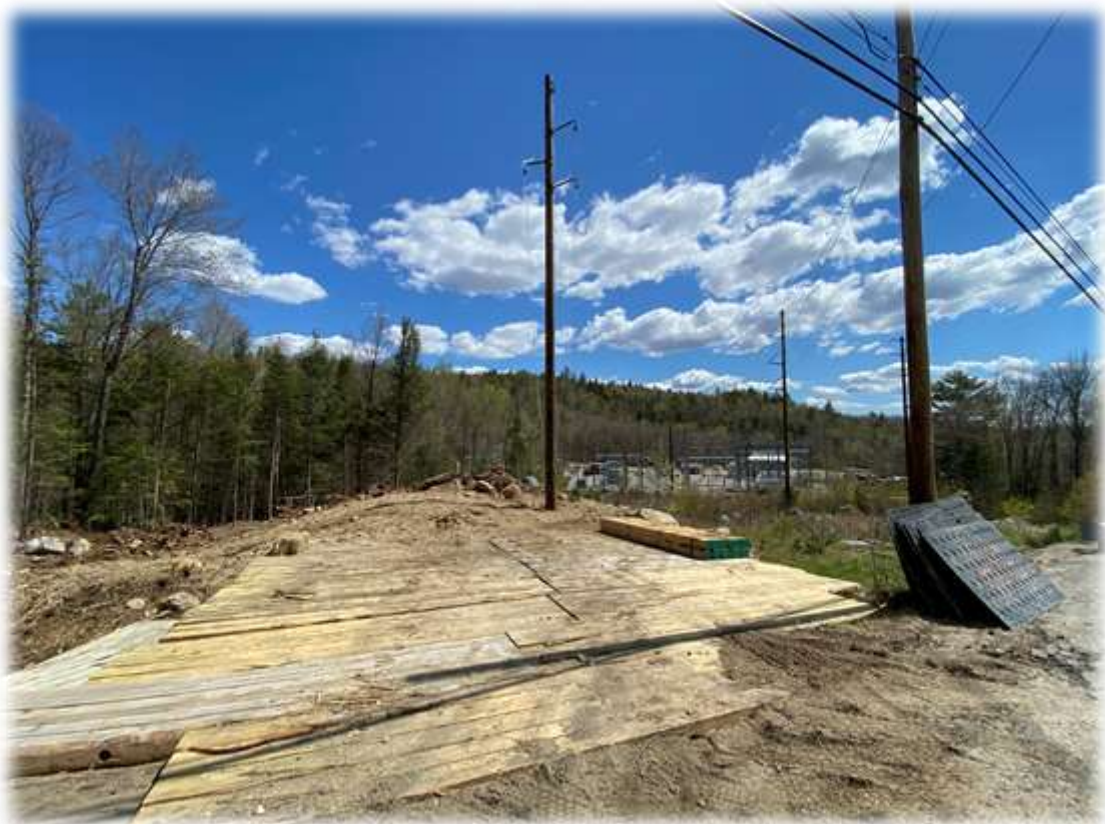
Photo #8: Structure 137-2 installed along Roxbury Road including structures adjacent to the substation.
