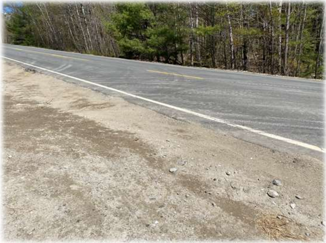
Photo #1: Roxbury Road pavement is clear of soil debris at the intersection with the SCADA building driveway.
