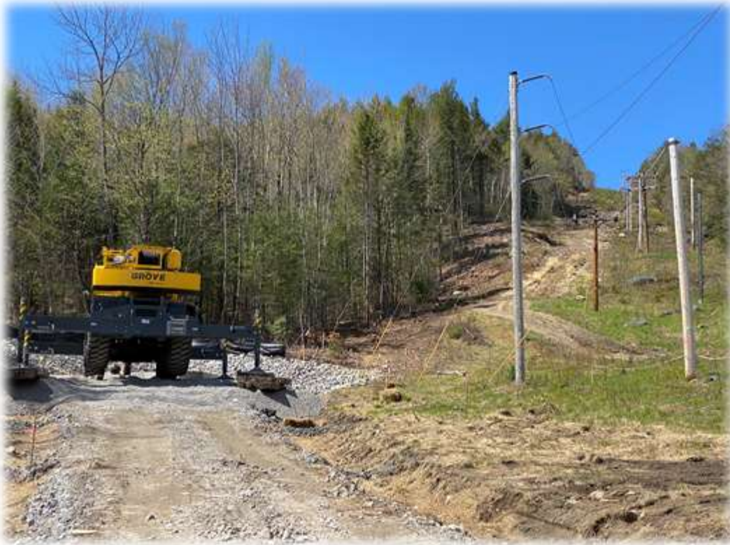
Photo #5: The gravel base material has been installed for the SCADA building driveway. Ditches have been cut and sideslopes heavily hay mulched. Temporary stone check dams have been placed until the fabric/riprap lining on the ditches can be installed. Riprap on fabric was placed along the upslope face of excavation.
