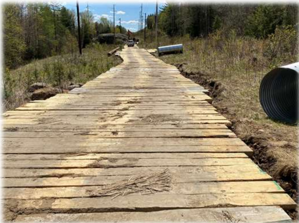
Photo #6: The view along the corridor (parallel with Roxbury Road) as seen from SCADA driveway. Structures have been laid-out. Matting installed to gain access to the structures in the area.
