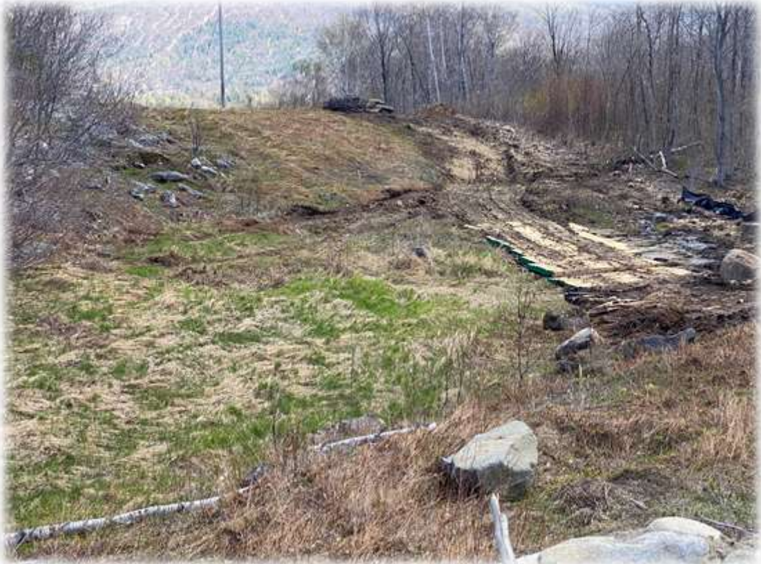
Photo #2: The upper portion of the transmission corridor coming into the RoxWind Towers portion of the project has been constructed. Mats have been installed in wetland areas.
