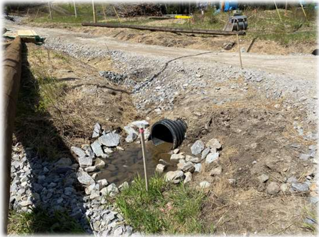
Photo #3: The riprap outlet plunge pool along the SCADA building driveway entrance has clear water within the pool.
