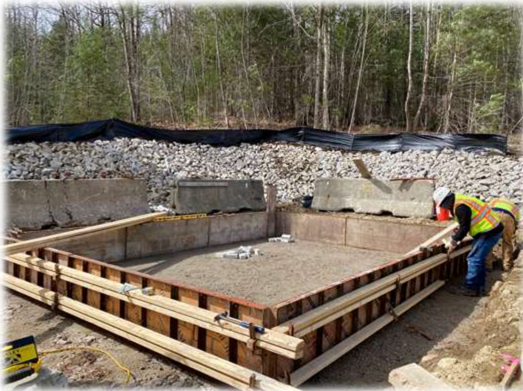
Photo #2: Sargent has completed excavation for the SCADA building and placed a gravel pad for forming the slab. Riprap on fabric was placed along the upslope face of excavation.
