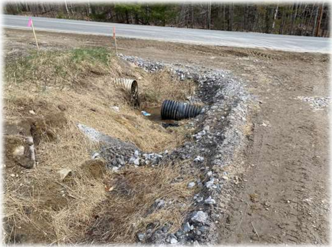
Photo #3: Riprap on fabric protection needs to be installed at the inlet/outlet to the driveway culvert at the entrance to Roxbury Road.
