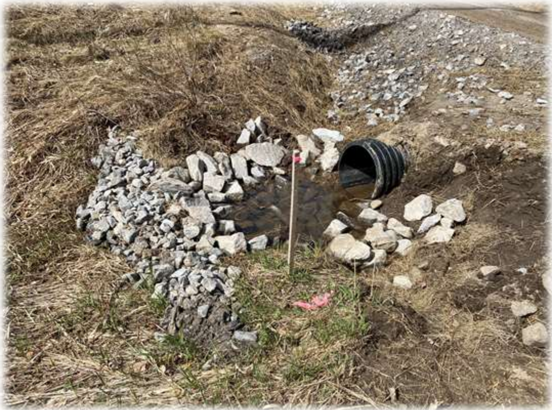
Photo #4: The driveway culvert outlet has clear water as it discharges towards a downslope stream.
