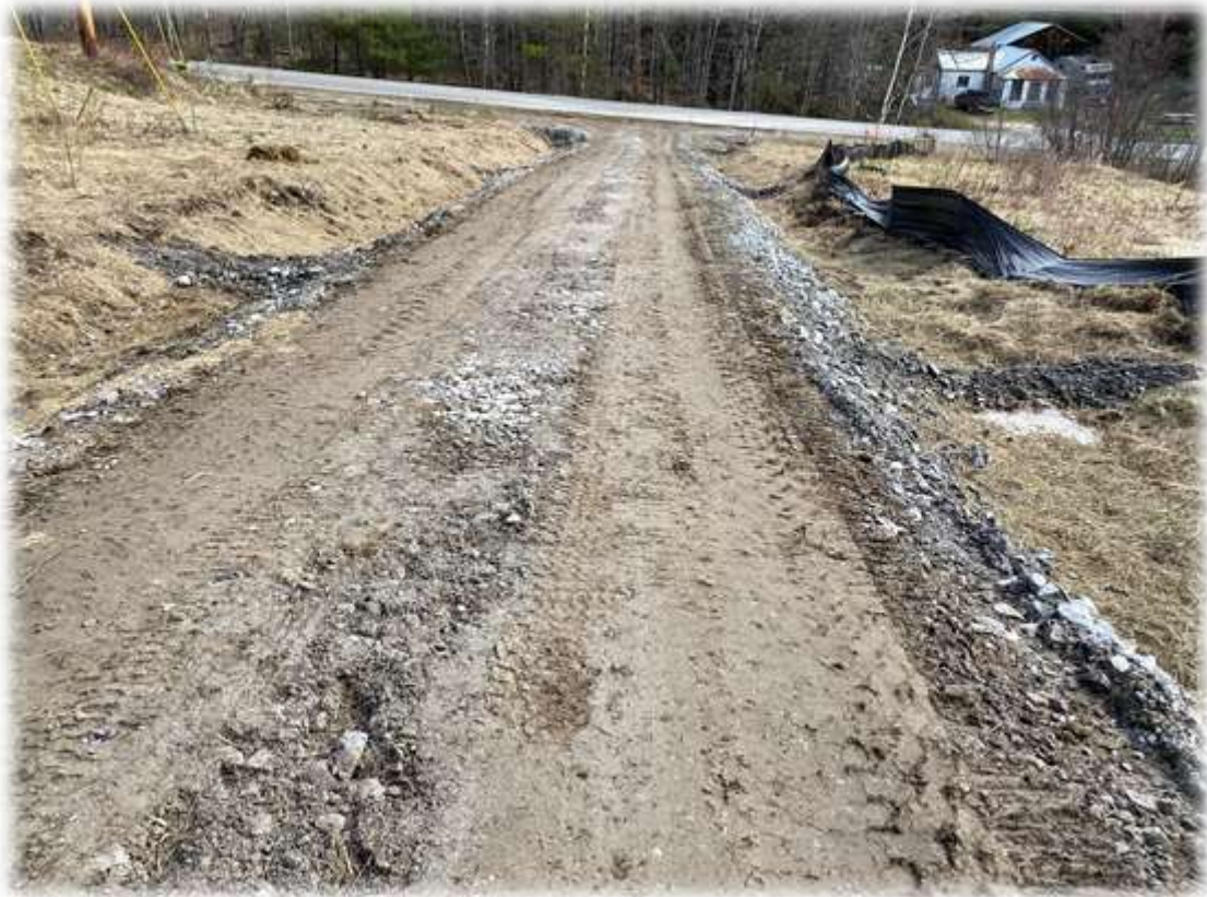
Photo #1: The gravel base material has been installed for the SCADA building driveway. Ditches have been cut and sideslopes heavily hay mulched. Temporary stone check dams have been placed until the fabric/riprap lining on the ditches can be installed.
