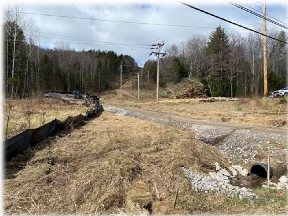
Photo #6: The view up the corridor as seen from Roxbury Road...No work has been performed along the corridor this construction season (too wet).
