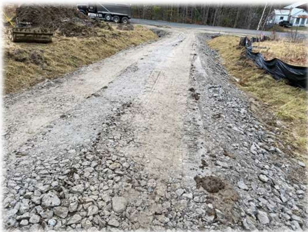
Photo #2: The gravel base material is being installed for the SCADA building driveway. Ditches have been cut and sideslopes heavily hay mulched. Temporary stone check dams have been placed until the fabric/riprap lining on the ditches can be installed.
