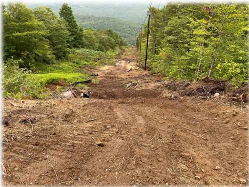
Photo #2: Water bars have been created along the corridor access road. The bars flow to a stabilized area with silt fence barrier to collect potential sediment wash
