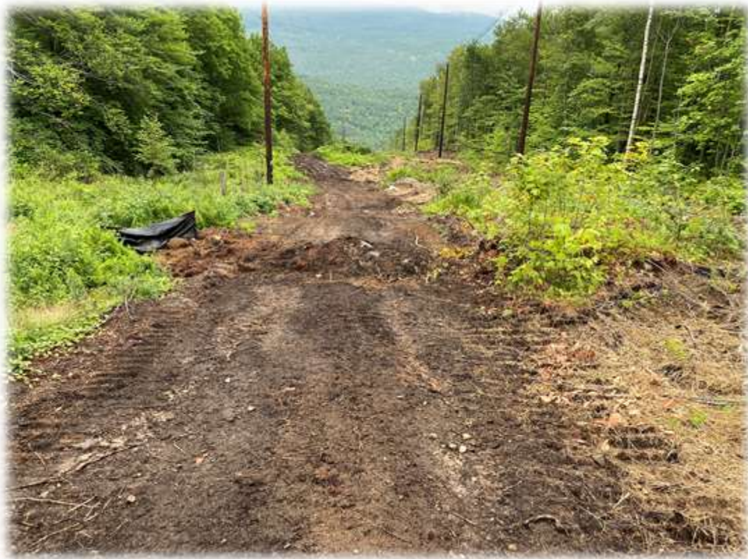
Photo #3: Water bars have been created to divert runoff water into stabilized areas.
