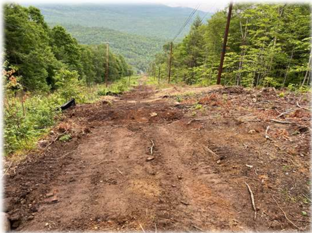
Photo #4: Water bars along the travel path have intercepted flows and diverted it into stabilized outlet areas.
