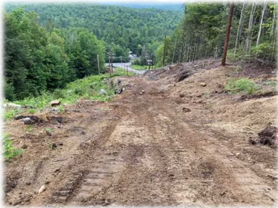
Photo #7: Water bars along the travel path have intercepted flows and diverted it into stabilized outlet areas. The water bars have been repaired (maintenance) and the collected sediment removed from the stabilized outlet.
