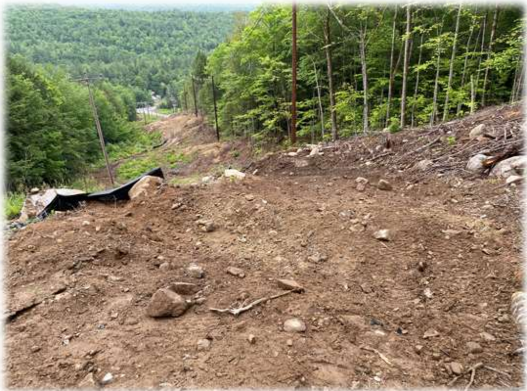
Photo #6: Water bars along the travel path have intercepted flows and diverted it into stabilized outlet areas. The water bars have been repaired (maintenance) and the collected sediment removed from the stabilized outlet.
