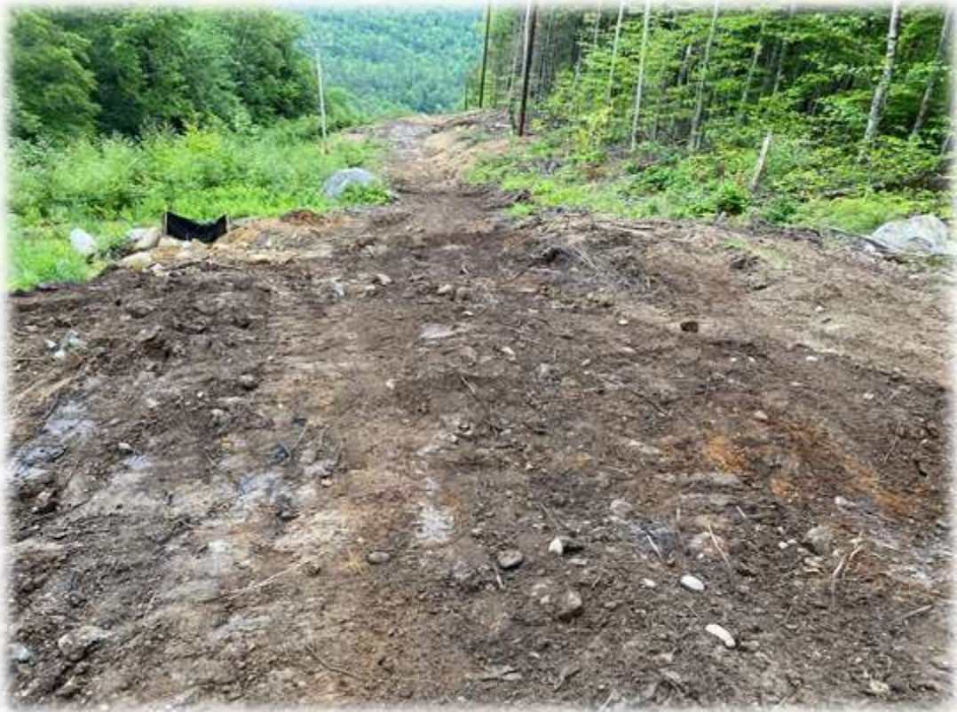
Photo #5: All water bars have been repaired (maintenance) and the collected sediment removed from the stabilized outlet.
