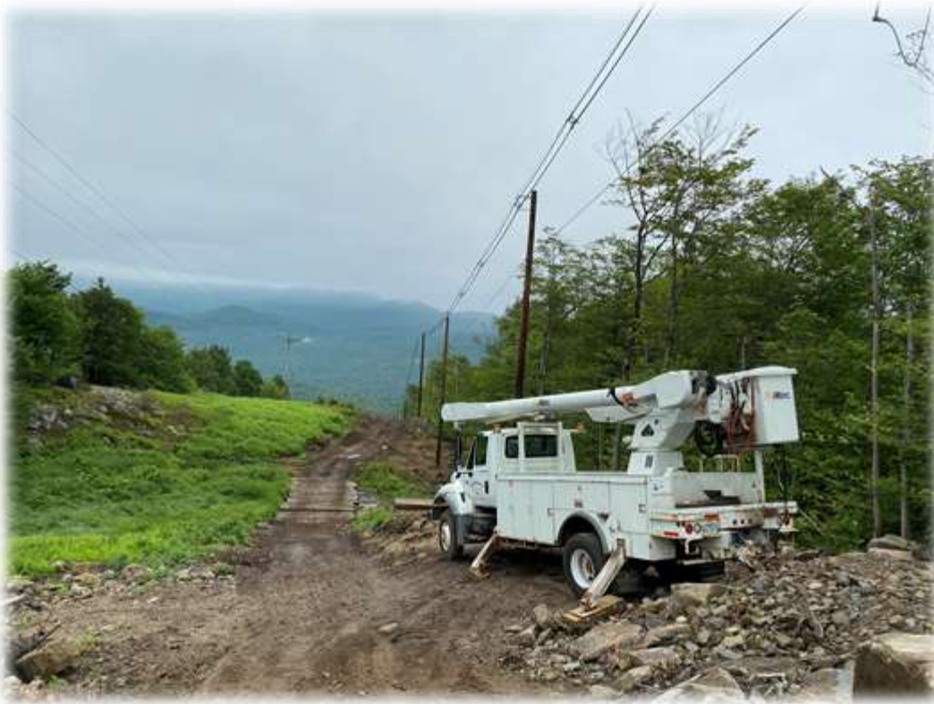
Photo #1: The upper portion of the transmission corridor access road coming into the RoxWind Towers portion of the project has been constructed and structures set. The corridor is damp and shows some areas of erosion along the travel path. The bars have captured and diverted these areas into stabilized areas.
