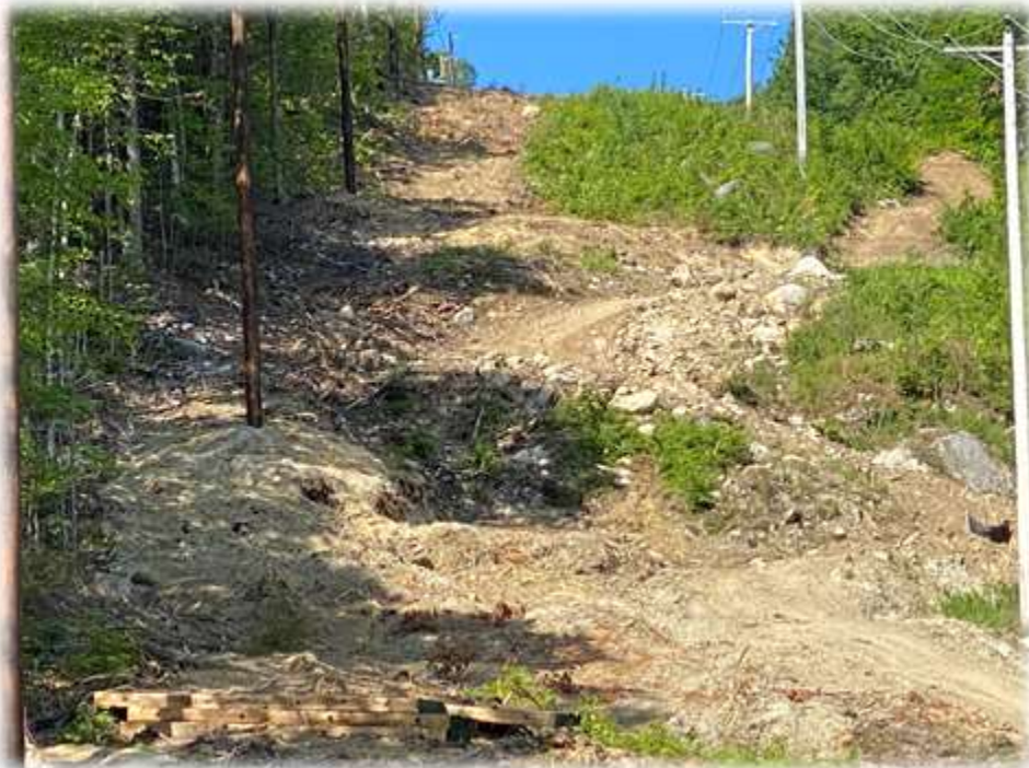
Photo #6: CLT has disturbed a new area adjacent to the woods line (near pole 18) that needs hay mulch.
