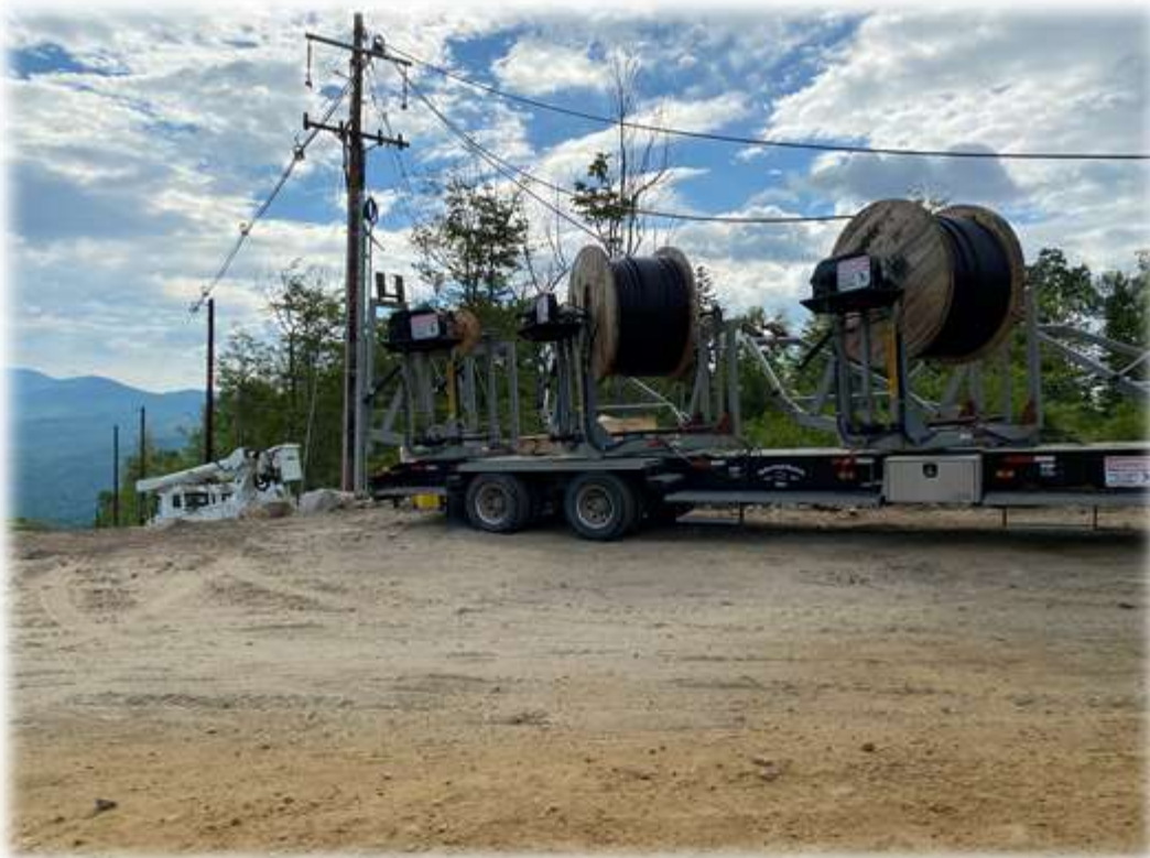
Photo #1: The upper portion of the transmission corridor access road coming into the RoxWind Towers portion of the project has been constructed and structures set. CLT has removed the "danger" trees from the corridor using hand labor and a forwarder. Underwood Electric has pulled ropes from top to bottom of the corridor.
