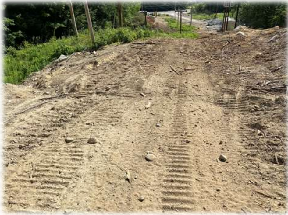
Photo #5: This area remains stable, but the water bars installed do not have any stabilized outlets. Sediments that are diverted by the bar will flow into vegetated areas and need to be removed.
