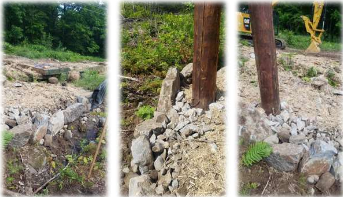
Photo #4: Structure P-23 has been placed along the side of a stream. Large rock has been placed in retaining wall formation with smaller stone inside the containment area. (Project generated photo from last week)
