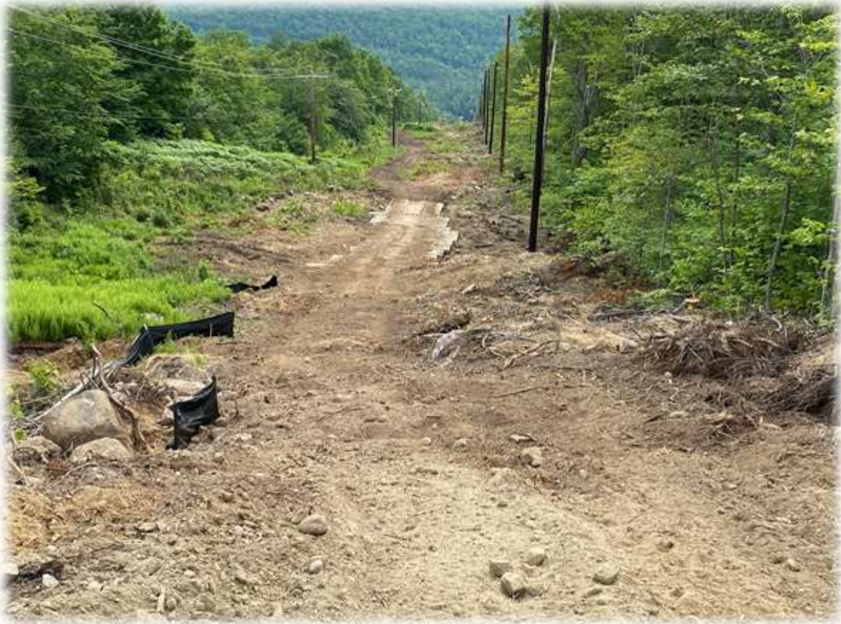
Photo #3: Water bars have been created along the corridor access road. The bars flow to a stabilized area with silt fence barrier to collect potential sediment wash
