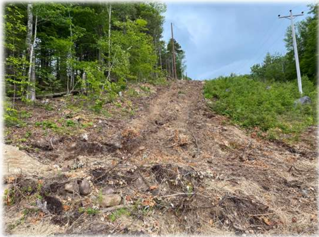
Photo #7: CLT has disturbed a new area adjacent to the woods line (near pole 18) that needs hay mulch (work in progress).
