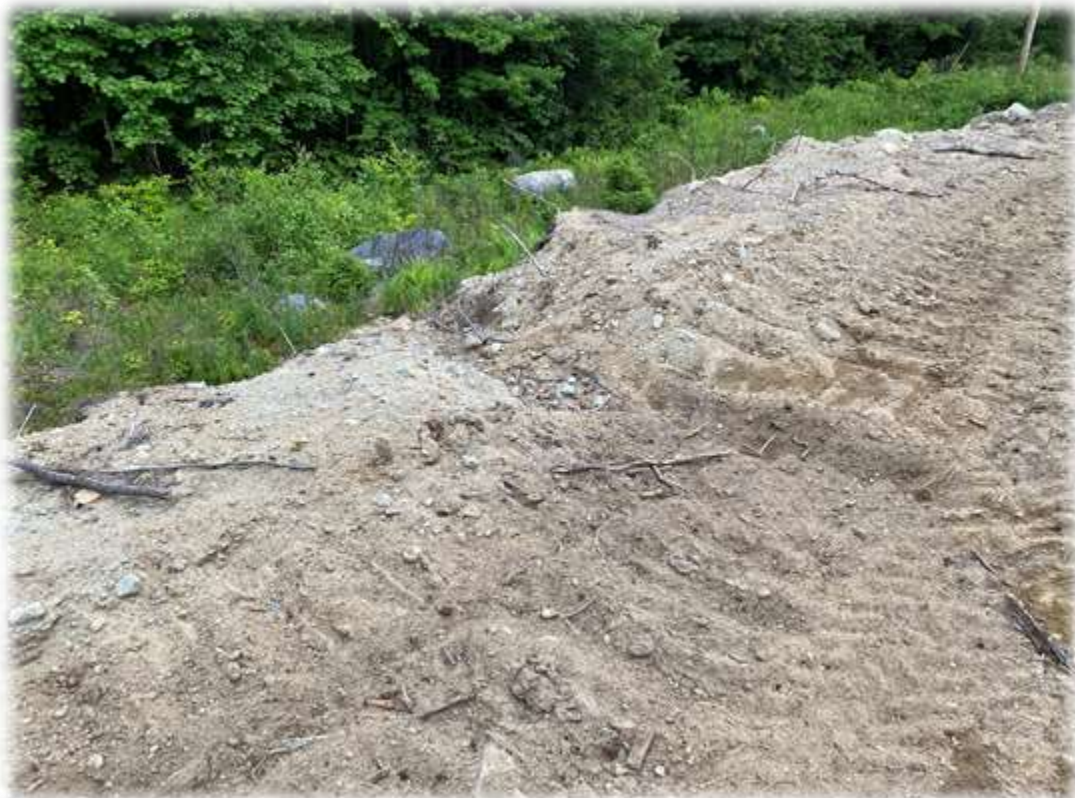
Photo #8: This area remains stable, but the water bars installed do not have any stabilized outlets. Sediments that are diverted by the bar will flow into vegetated areas and need to be removed.
