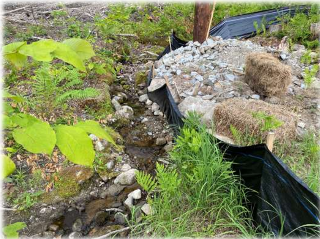
Photo #4: Structure P-23 has been placed along the side of a stream. Silt fence and rock have been placed to minimize impact to the stream. Some of the rock that has fallen into the stream has been removed. No action has been taken regarding removing the silt fence and resulting rock fall into the stream.
