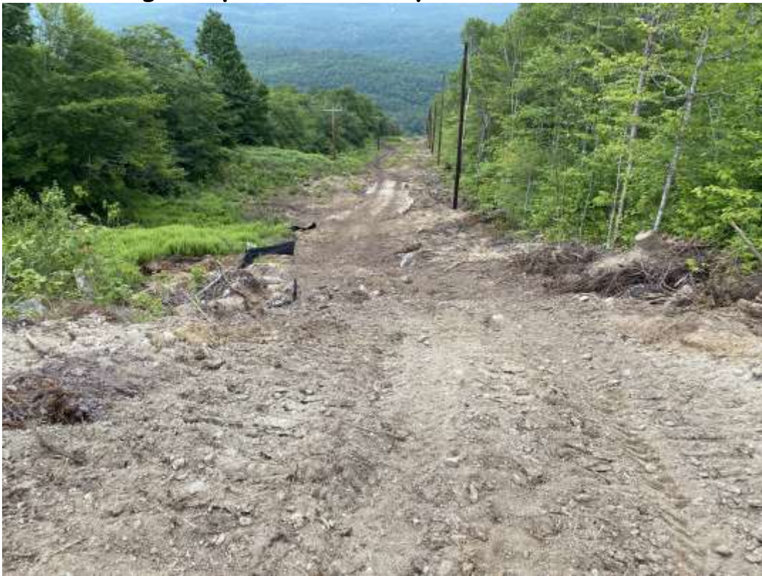
Photo #1: The upper portion of the transmission corridor access road coming into the RoxWind Towers portion of the project has been constructed and structures set. CLT has removed the "danger" trees from the corridor using hand labor and a forwarder. They have re-constructed most of the water bars.
