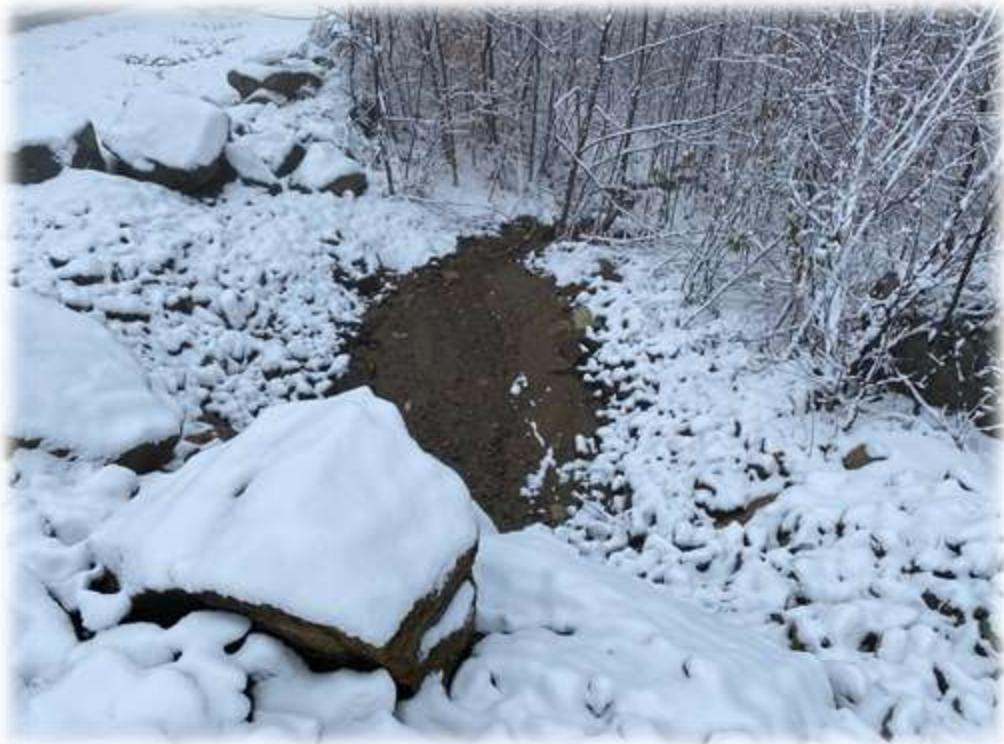
Photo #6: Outside view of same culvert (sta 124+50) showing washed gravel flowing in stream.
