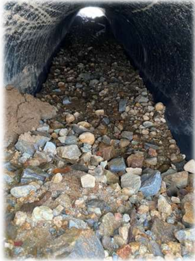
Photo #5: The new gravel fill inside the stream culverts has washed fines from the soil by this weekend's significant rain event.
