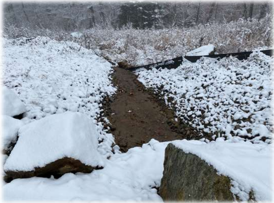
Photo #3: Some soil material within the \frac{1}{2} filled stream culvert has washed and has been captured by the silt fence.
