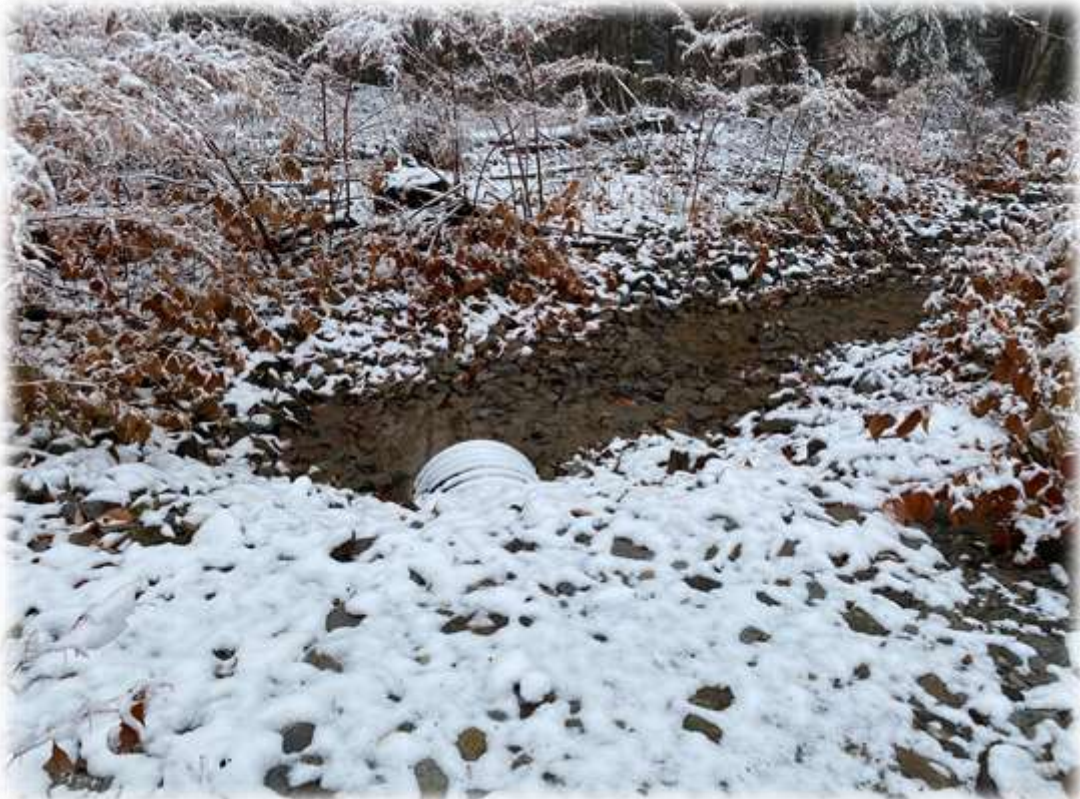
Photo #2: Sediment within the rocky plunge pool area across from the driveway entrance has been removed. No significant new sediment buildup noted. Water in pool is slightly turbid.
