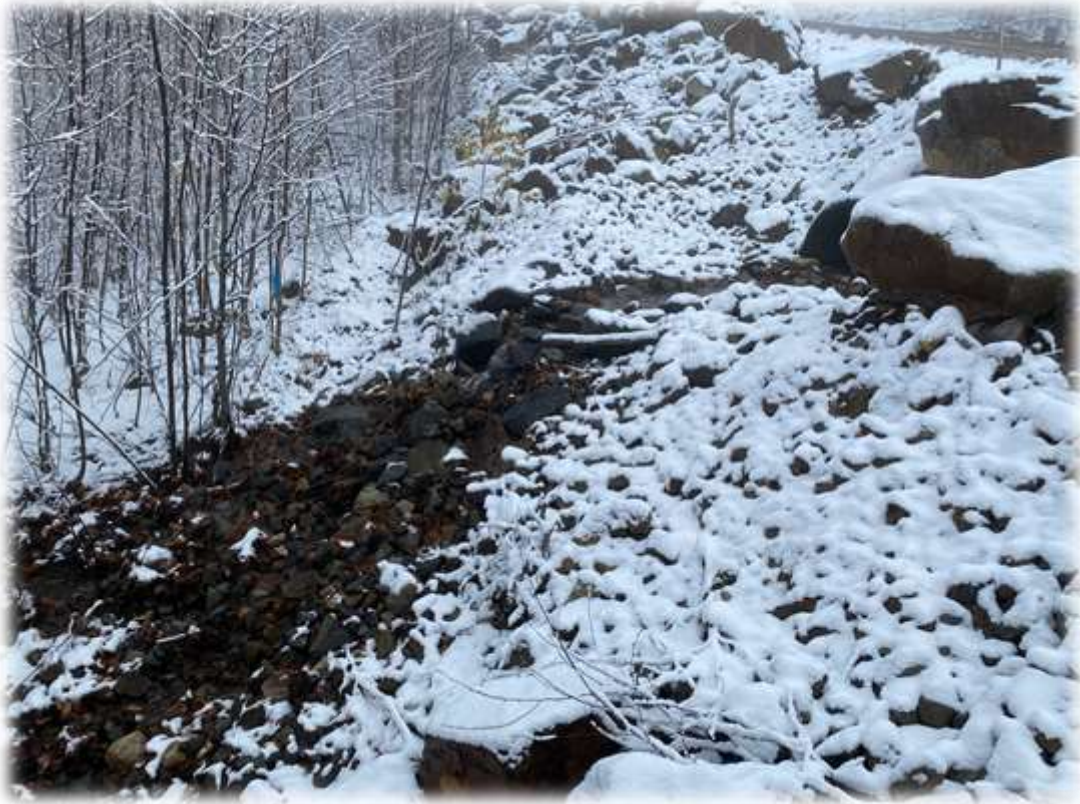
Photo #7: While the picture does not reflect the vertical elevation very well (8' drop), the discharge end of culvert at sta 125+50 has significant riprap on fabric protection that distributes the concentrated pipe flow over the whole rock.
