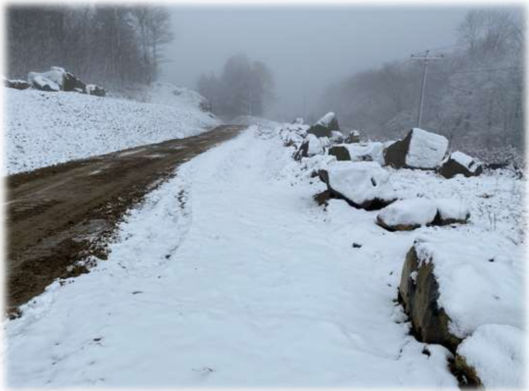
Photo #4: Snow cover in the filter media ditch construction along the main access road depicts some areas that the filter media has eroded. Sargent is repairing these locations along the bottom \frac{1}{2} mile of main access road.
