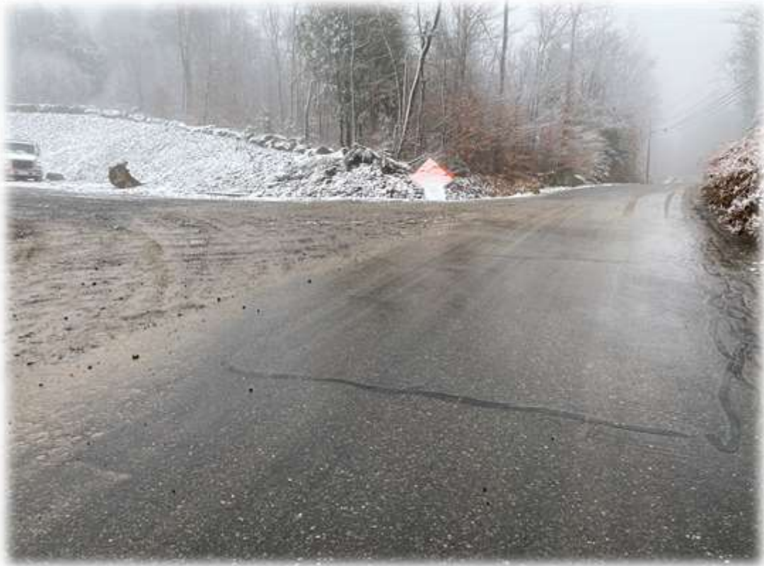
Photo #1: The Contractor has removed crushed stone from the Horseshoe Valley Road intersection with the project driveway. A slight covering of silt material is being tracked onto the paved surface that should be removed periodically throughout the day at this time of year.
