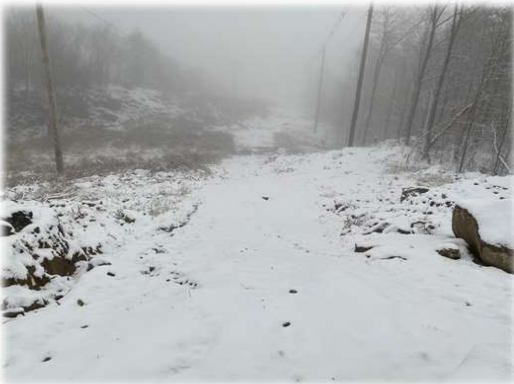
Photo #10: The upper portion of the transmission corridor access road coming into the RoxWind Towers portion of the project has been restored. Water bars have captured and diverted upland areas into stabilized areas. A significant catch of vegetation is becoming established. Some erosion is beginning to occur that should be redirected at the rock barrier along the road.
