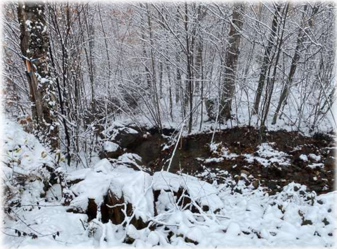
Photo #8: The stream along the downslope side of culvert 125+50 is relatively clear water.
