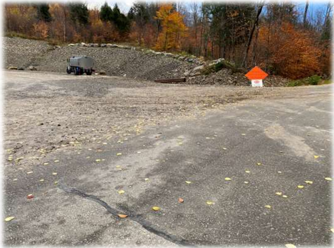
Photo #1: The Contractor has removed crushed stone from the Horseshoe Valley Road intersection with the project driveway. A slight covering of sand material is being tracked onto the paved surface that should be removed daily at this time of year.
