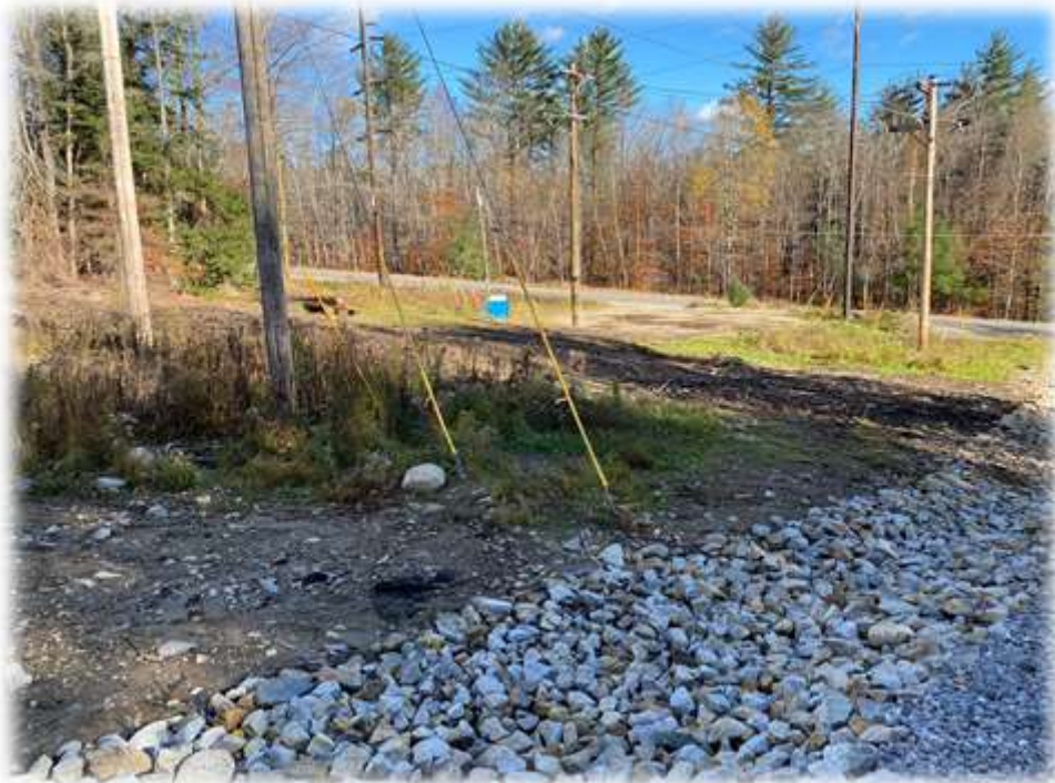
Photo #12: The laydown area at the bottom of the corridor needs additional seed/mulch for a better vegetative catch.
