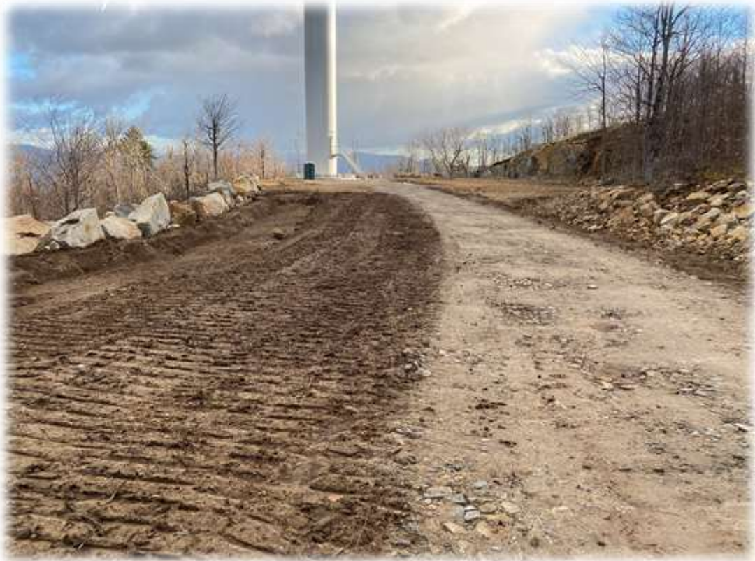
Photo #9: The Contractor has restored and loamed Tower 2 area and has created a filter media ditch along the downslope side of access road. The site is partially hydroseeded and mulched. No erosion has been noted.
