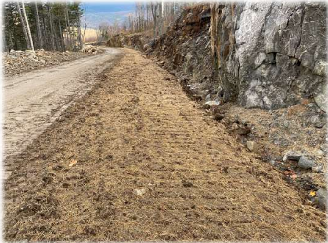
Photo #6: The loam/seed/mulch material has been applied to the restored access road between Towers 2/3. No erosion issues have been noted.
