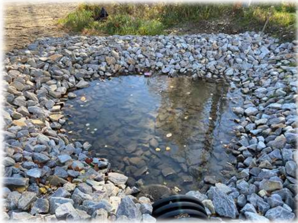
Photo #11: The culvert plunge pool along the SCADA building driveway has clear water within the pool.
