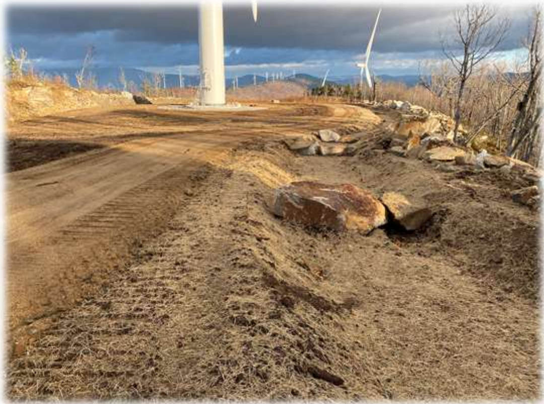
Photo #7: The access road has been made narrower (12' wide) and the remaining area loamed and tracked in near tower 3. The Tower 3 area is partially hydroseeded.
