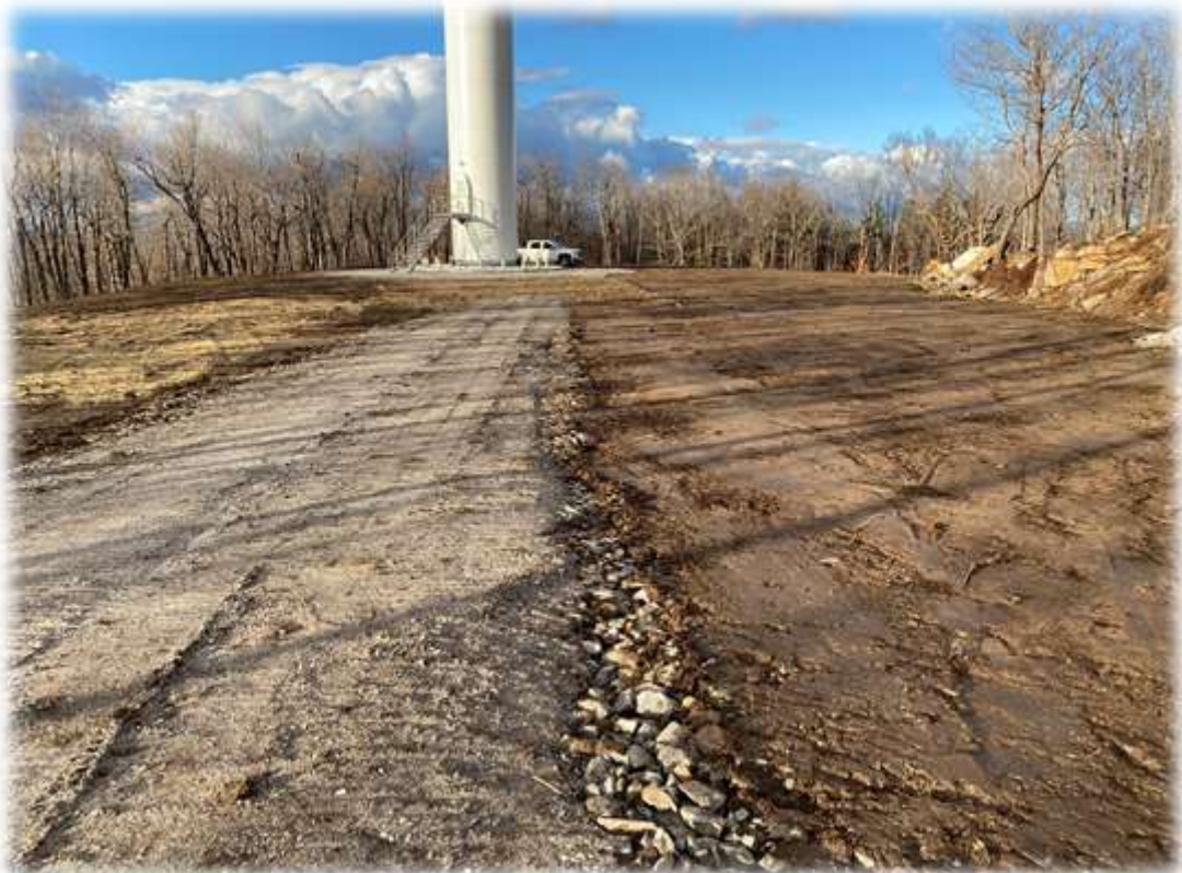
Photo #8: The access road has been made narrower (12' wide) and the remaining area loamed and tracked in near tower 4. The Tower 4 area is partially hydroseeded.
