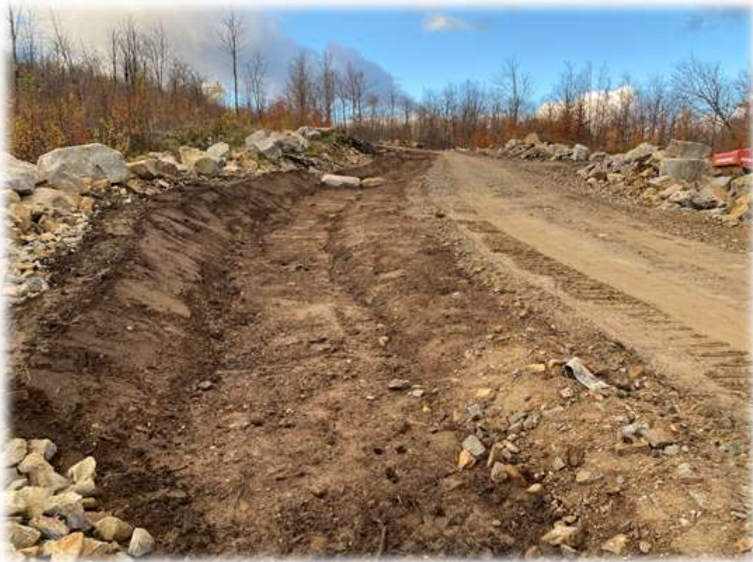
Photo #5: The Contractor continues restoring the narrower access road and has constructed the filter media ditch along the left side of access road. They have constructed to the 180 degree road curve near tower 1 to tower 4. No erosion or ponding of water was noted in the filter media ditch.
