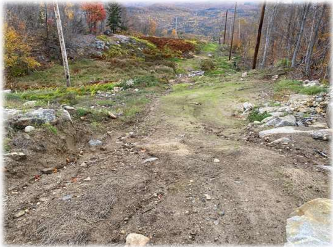
Photo #5: The upper portion of the transmission corridor access road coming into the RoxWind Towers portion of the project has been restored. Water bars have captured and diverted upland areas into stabilized areas. A significant catch of vegetation is becoming established. Some erosion is beginning to occur that should be redirected at the rock barrier along the road.
