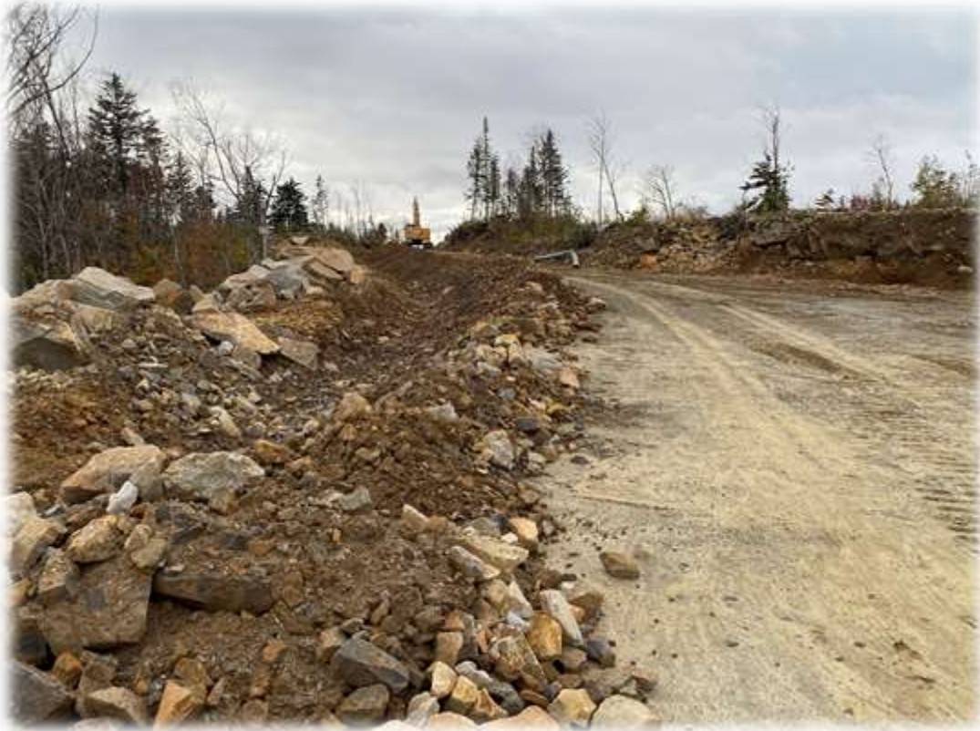
Photo #9: The Contractor is creating new riprap ditches and restoring the access road between Towers 3 and 4.
