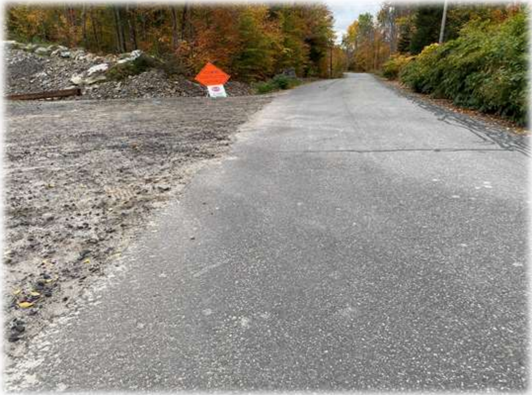
Photo #1: The Contractor has removed crushed stone from the Horseshoe Valley Road intersection with the project driveway.
