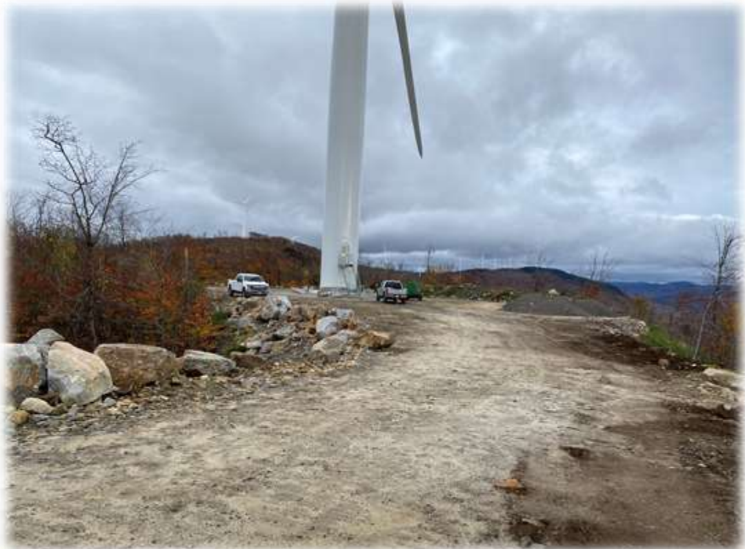
Photo #6: Final gravel is being stockpiled for use in constructing Tower 1 base padsite.
