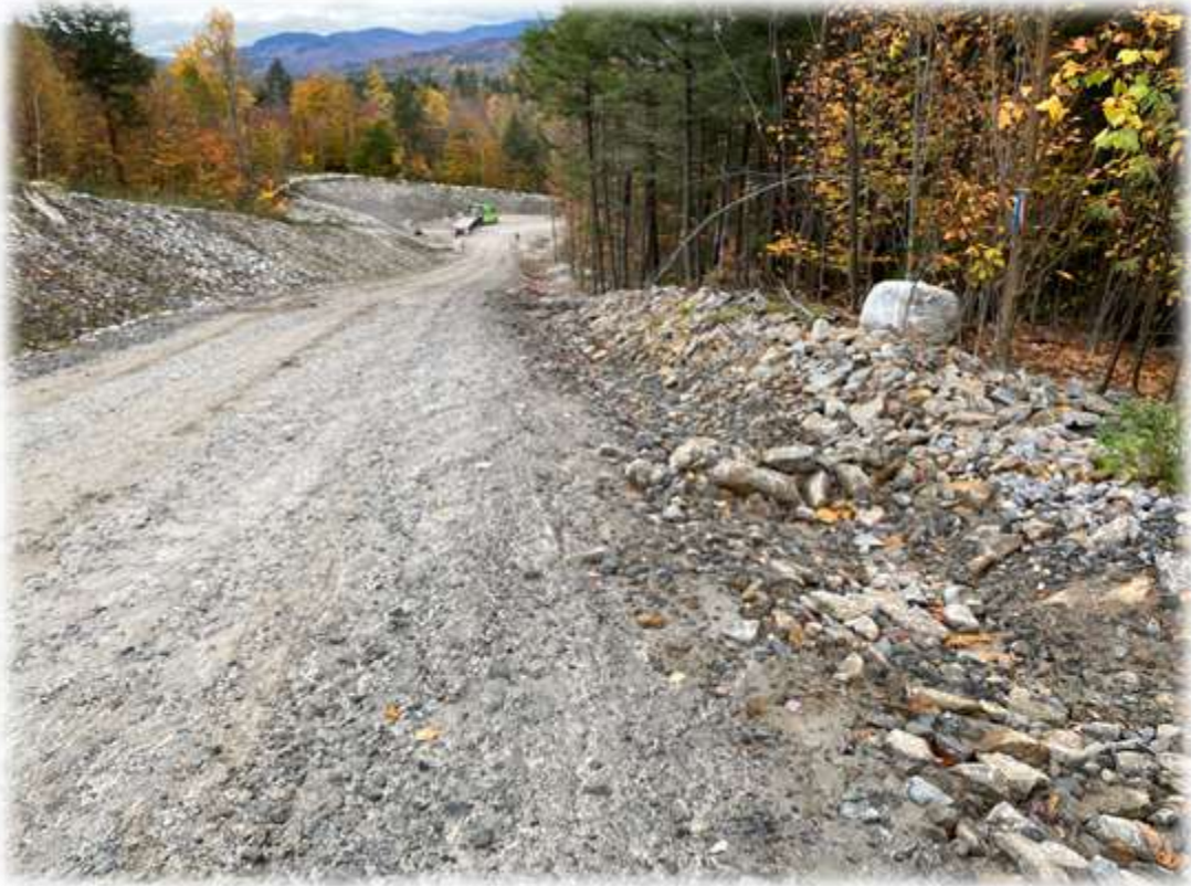
Photo #3: Sediment has been removed from the stone check dams along the first hill of the tower access road.
