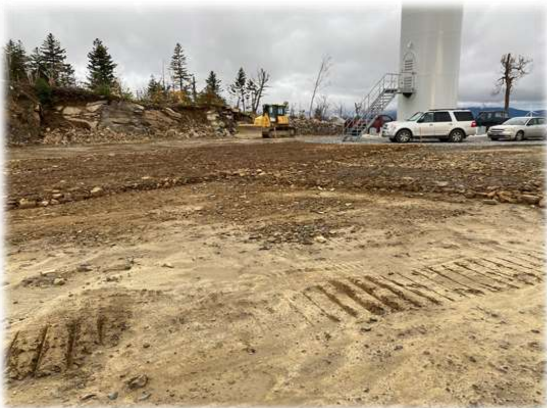
Photo #8: Ongoing testing operations at Tower 2 location. The Contractor is constructing the tower base padsite area.
