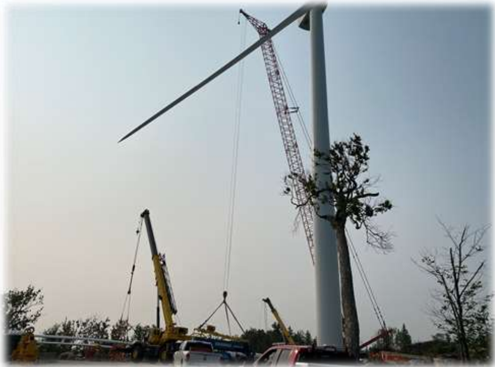
Photo #6: The base, mid-section top section, hub, and 1 blade of Tower 3 have been set.
