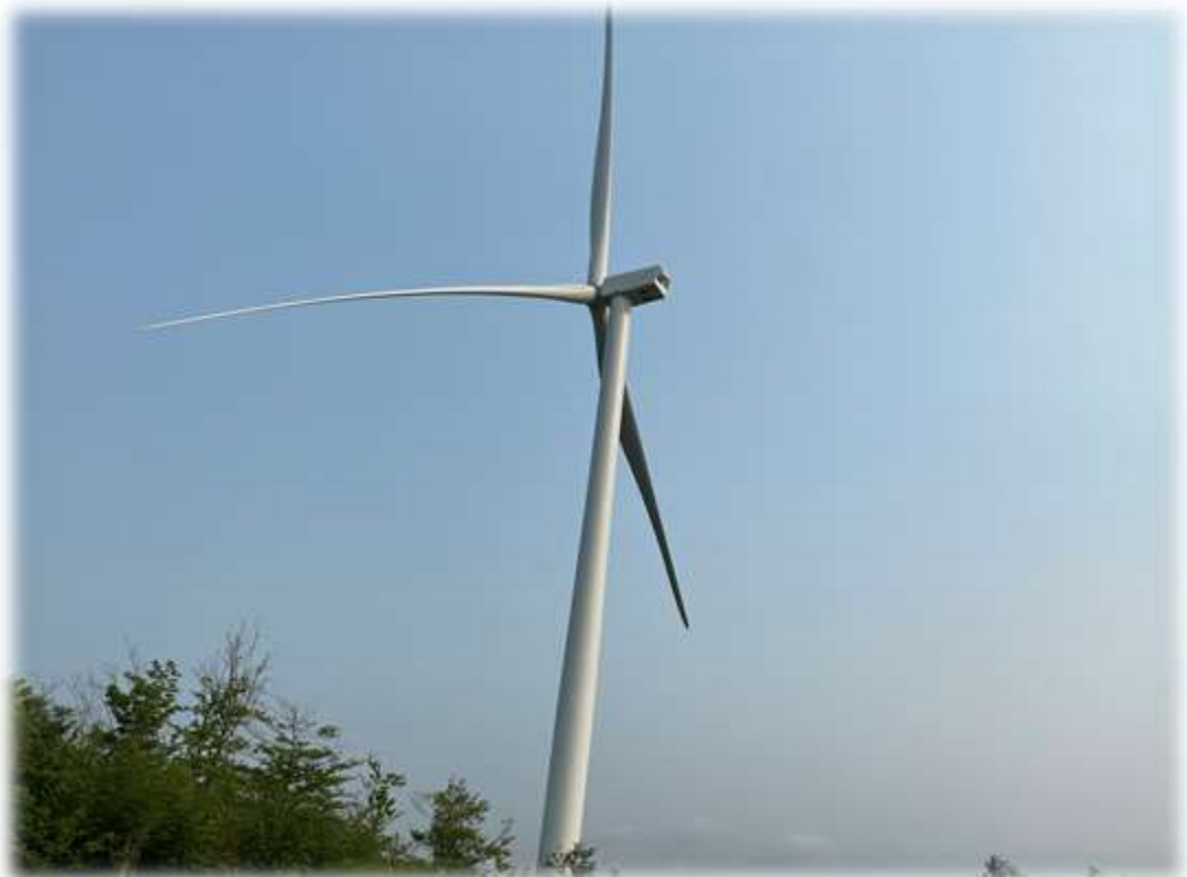
Photo #4: Tower 1 has been set including the Nacelle, blade hub, and 3 blades at the top of the tower.
