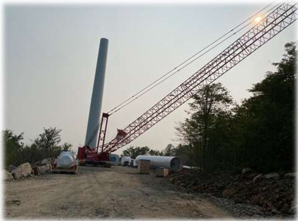
Photo #5: The base and mid-section of Tower 2 has been set. No changes to this padsite have occurred in this area this past week.
