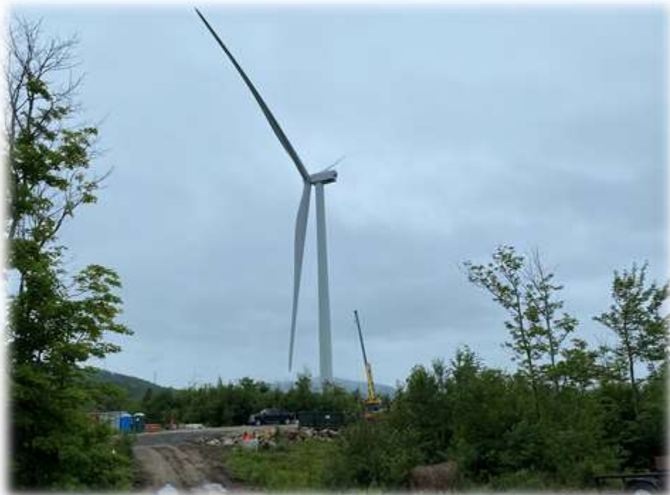
Photo #6: Tower 1 has been set including the Nacelle, blade hub, and 3 blades at the top of the tower. The crane has been taken apart and is being reassembled at tower 4.
