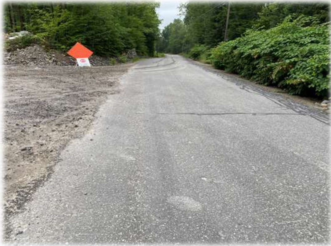
Photo #1: Horseshoe Valley Road is clear of soil debris.
