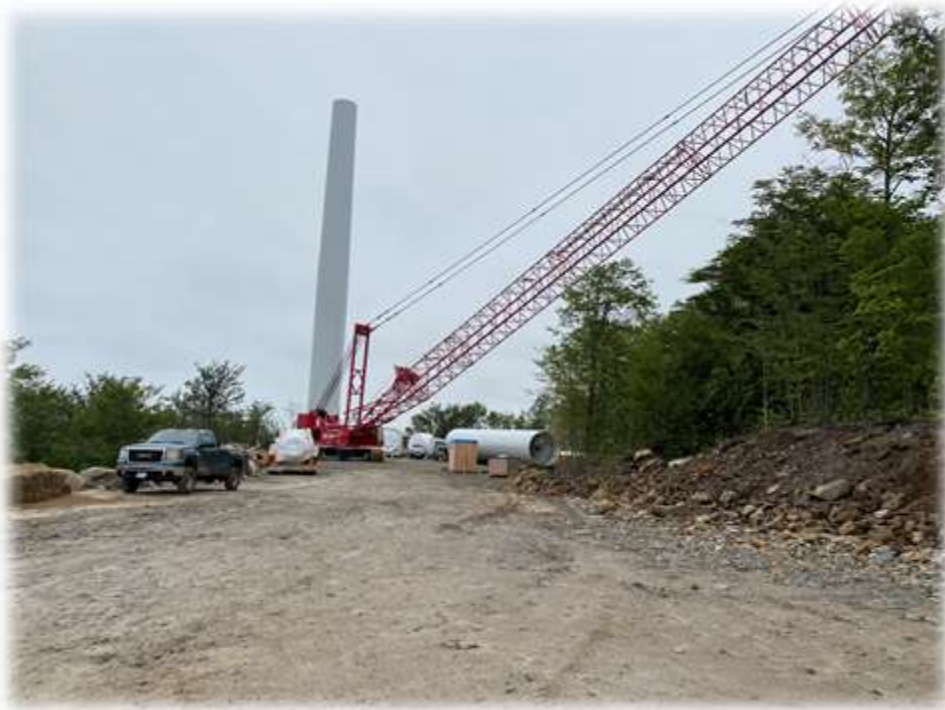
Photo #5: The base and mid-section of Tower 2 has been set. Reed/Reed crane is mobilized for future work in this area.
