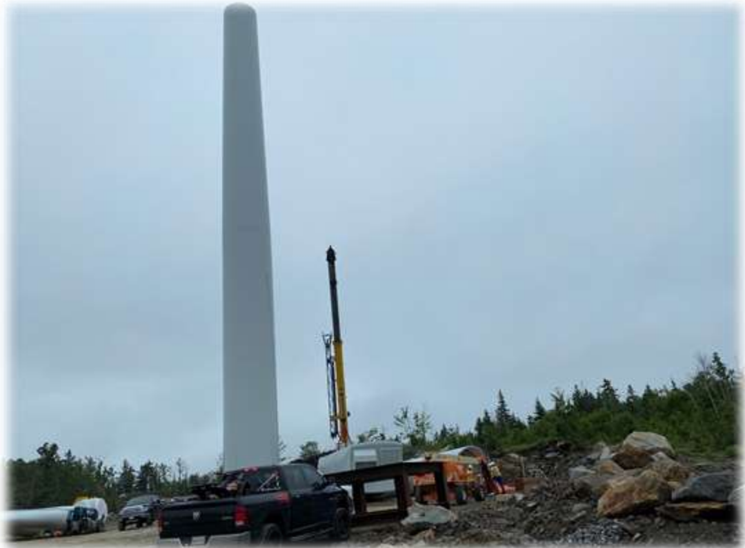
Photo #4: The base and mid-section of Tower 3 has been set. No significant changes since last week. Contractor is prepping site for crane reassembly.
