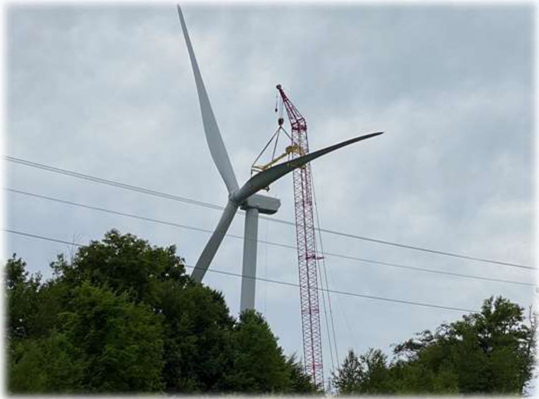
Photo #7: Tower 1 has been set including the Nacelle, blade hub, and 3 blades at the top of the tower.
