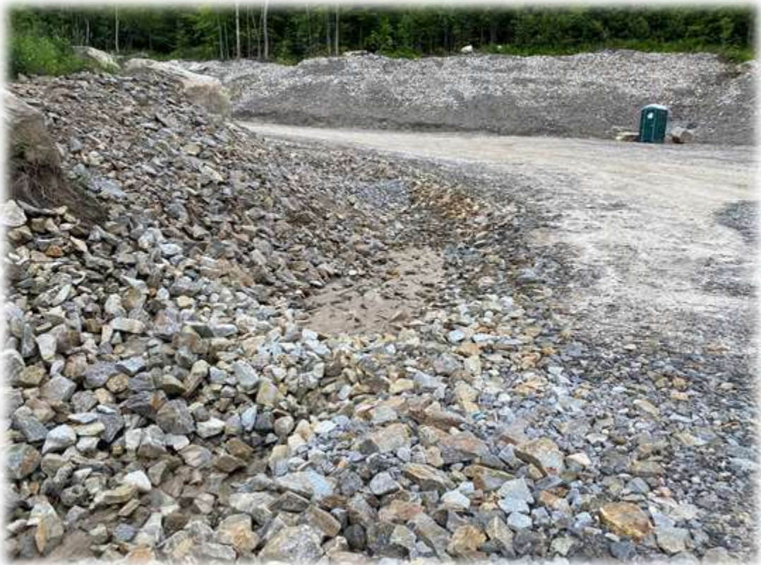
Photo #4: Stone berms within the riprap road ditches have captured some soil material.
