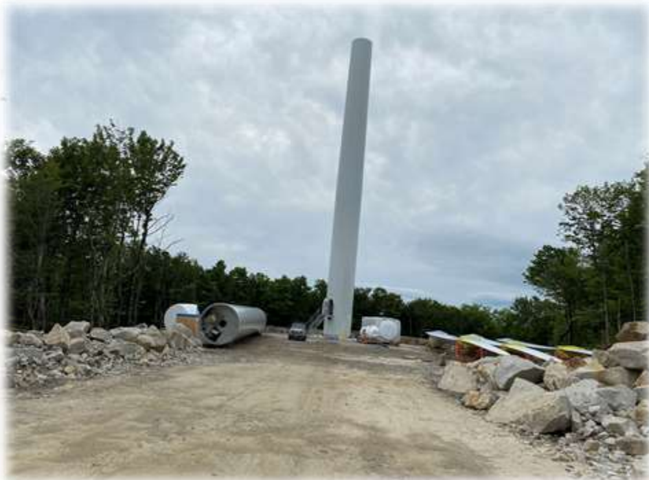
Photo #10: The base and mid-section of Tower 4 has been set. No significant changes since last week.
