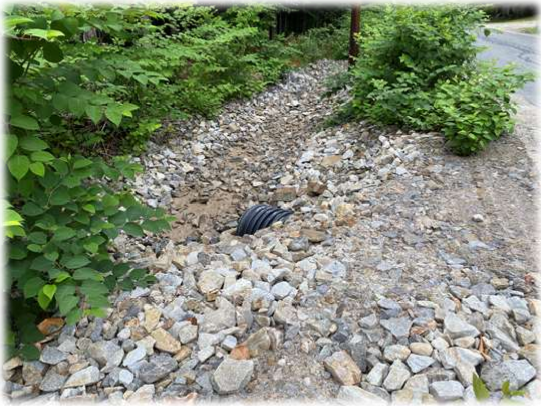
Photo #3: The drainage ditch across Horseshoe Valley Road has no water...
