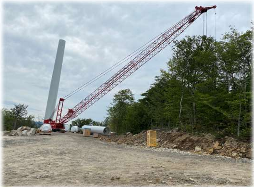
Photo #8: The base and mid-section of Tower 2 has been set. Reed/Reed crane is mobilized for future work in this area.
