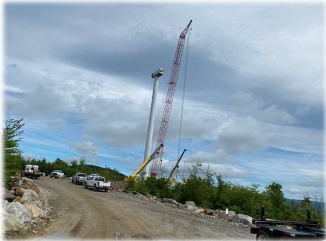
Photo #4: Tower 1 has been set including the Nacelle and blade hub at the top of the tower. Crews were preparing to lift the first blade for attachment to the hub until the wind started blowing.
