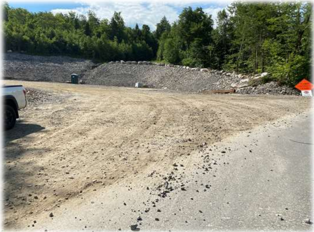
Photo #2: The stabilized construction entrance needs new stone re-installed.
