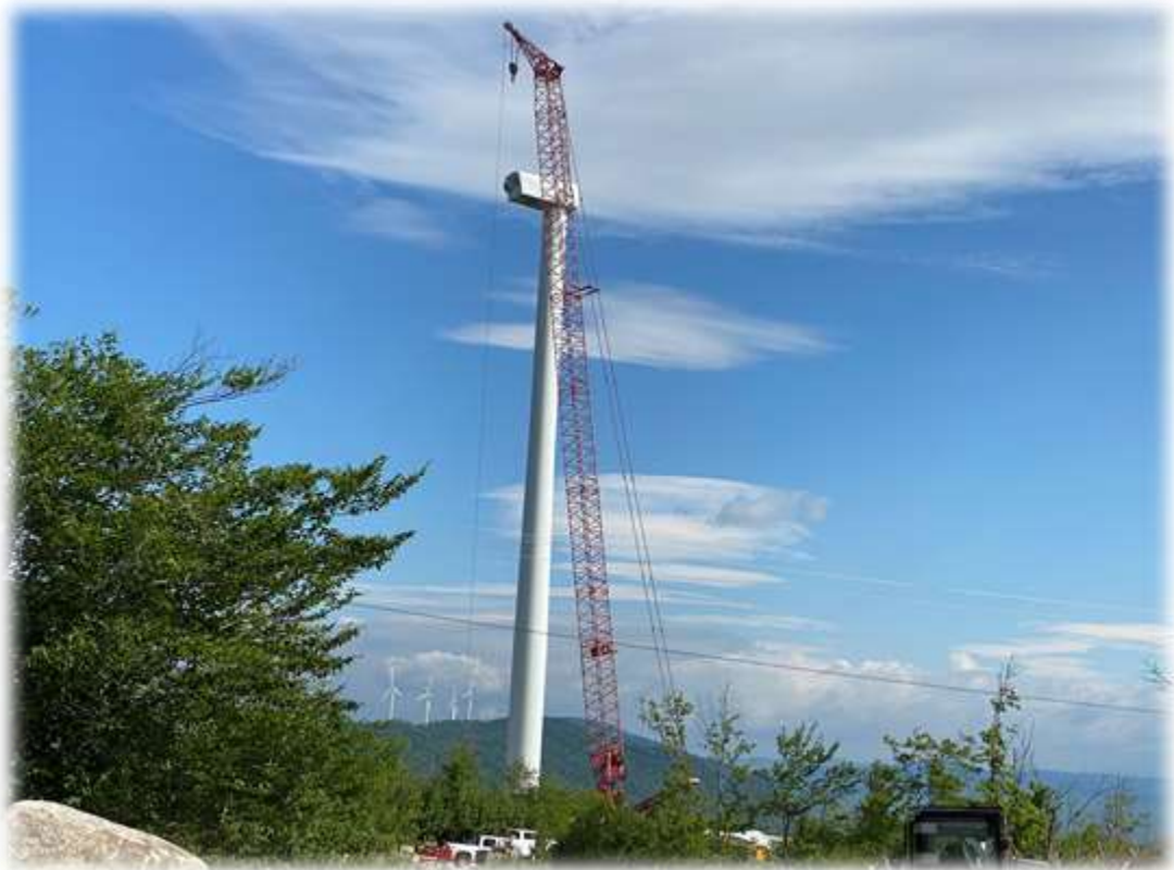
Photo #4: Tower 1 has been set including the Nacelle at the top of the tower.
