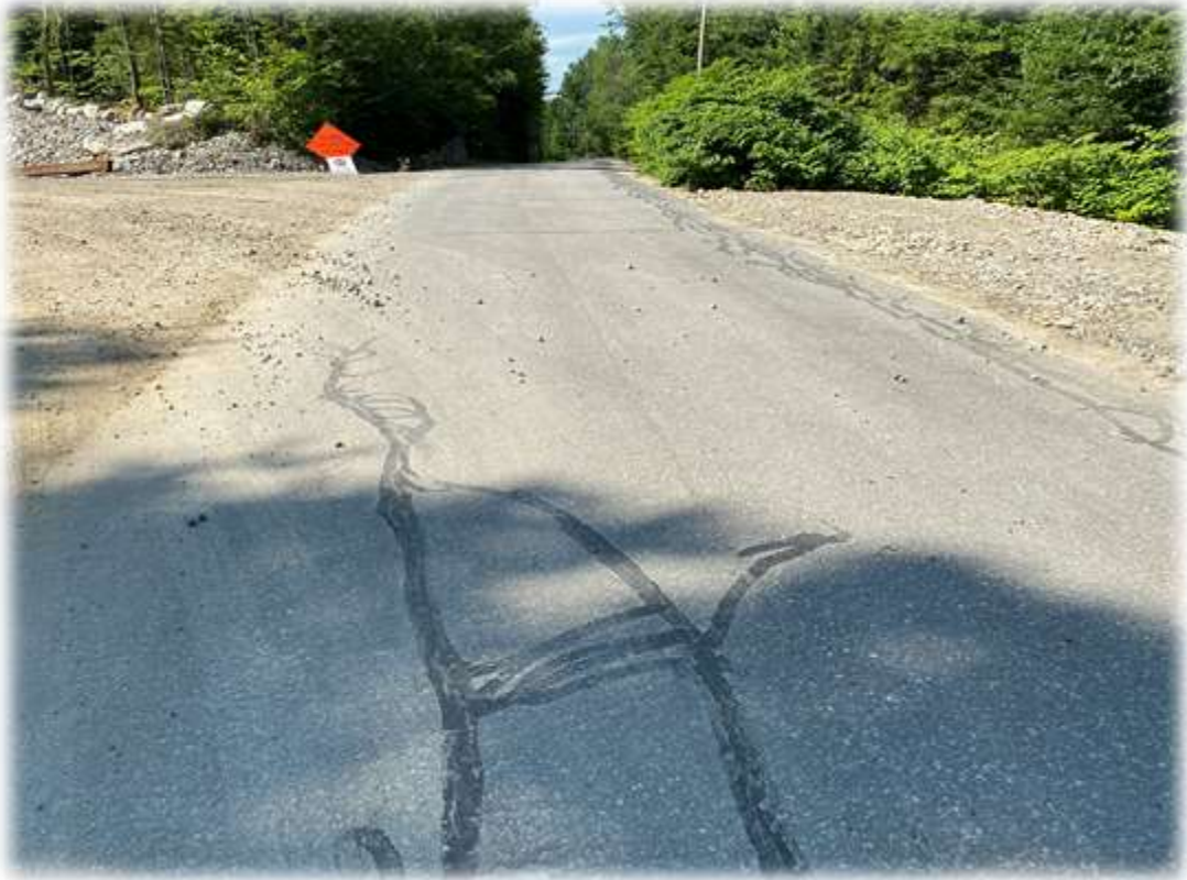
Photo #1: Stone is creeping out into Horseshoe Valley Road and needs to be removed.
