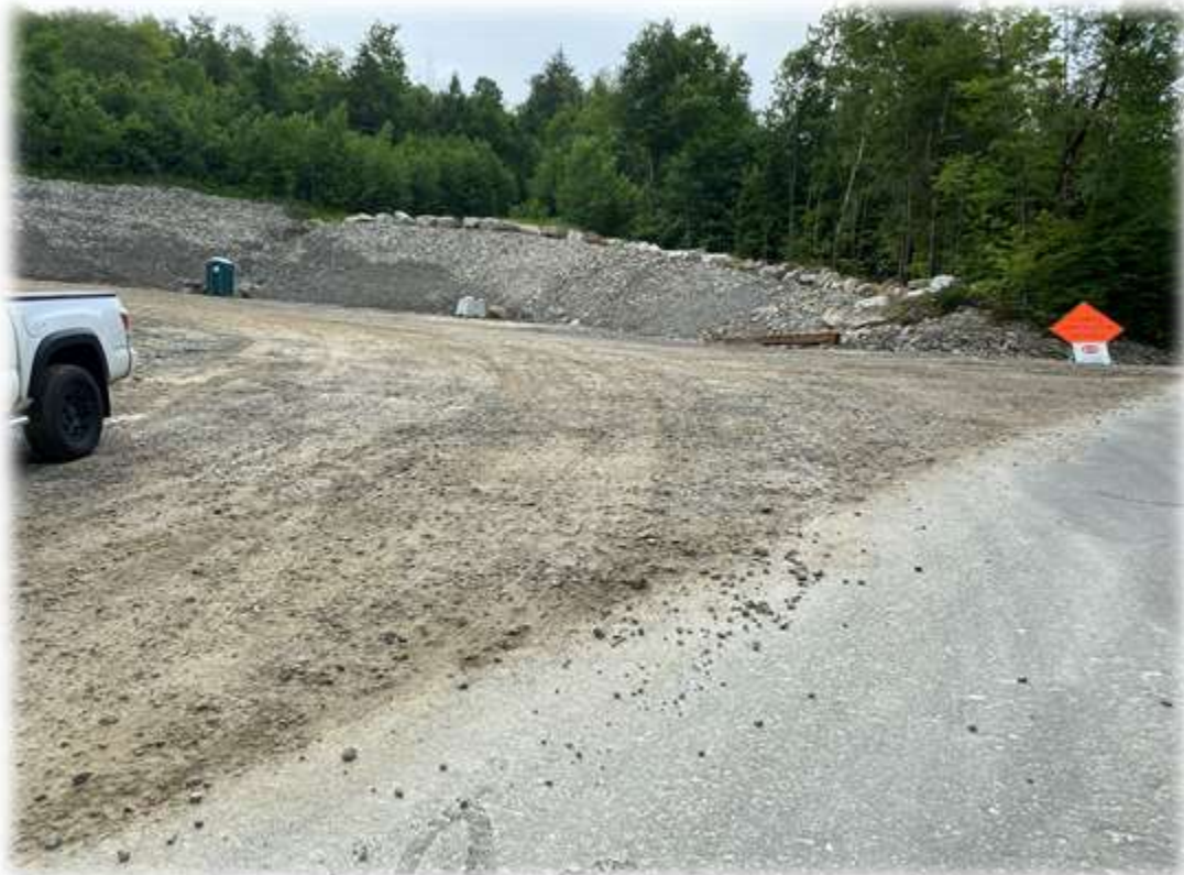
Photo #2: The stabilized construction entrance been removed in order to bring tower sections and blades into the project. There is no debris being transported onto Horse Valley Road.
