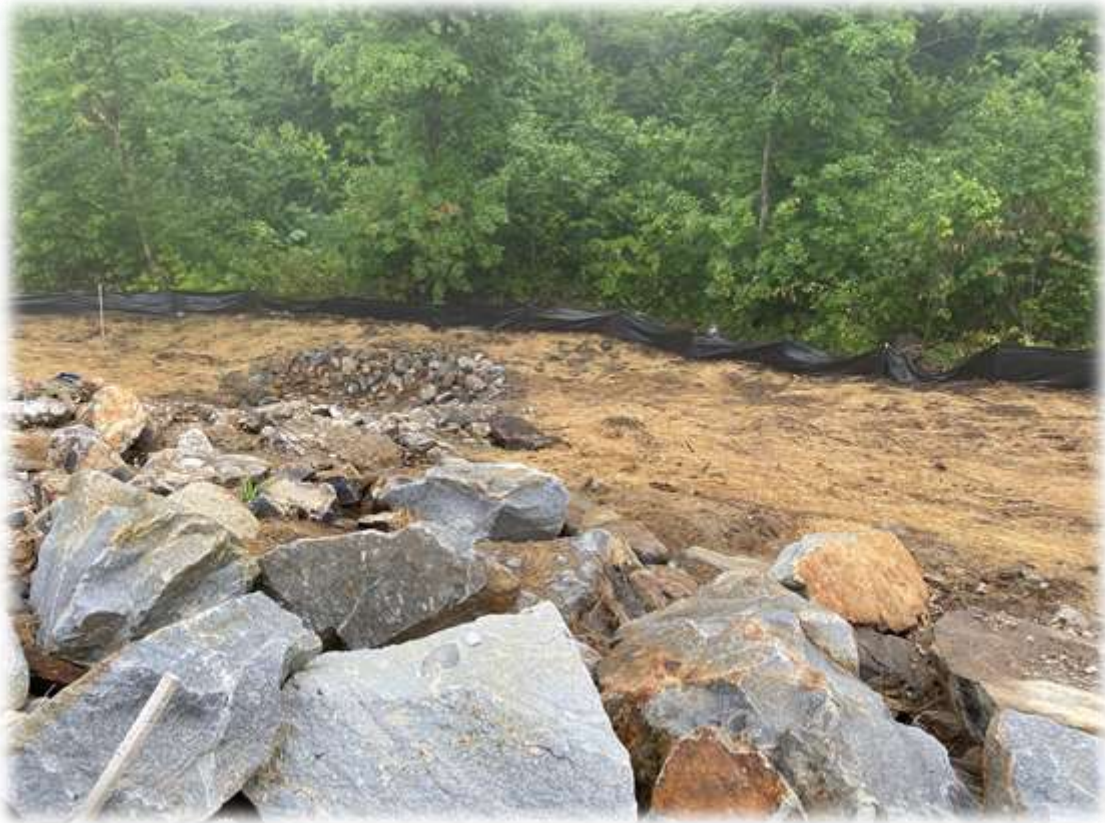
Photo #5: The former silt fence between Tower 1 and the corridor has been removed, the area cleaned of collected sediment, and new silt fence installed. Disturbed areas have been mulched.
