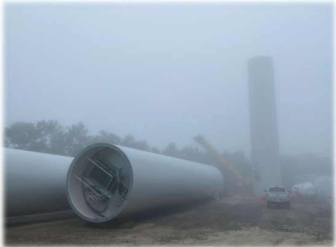
Photo #4: The base section of Tower 4 has been set. All of the tower sections have been delivered to the site. Many of the blades have been delivered to the site.
