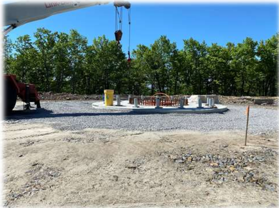
Photo #6: No significant earthwork is ongoing at the tower portion of the project. Backfill at Tower 4 has been completed.
