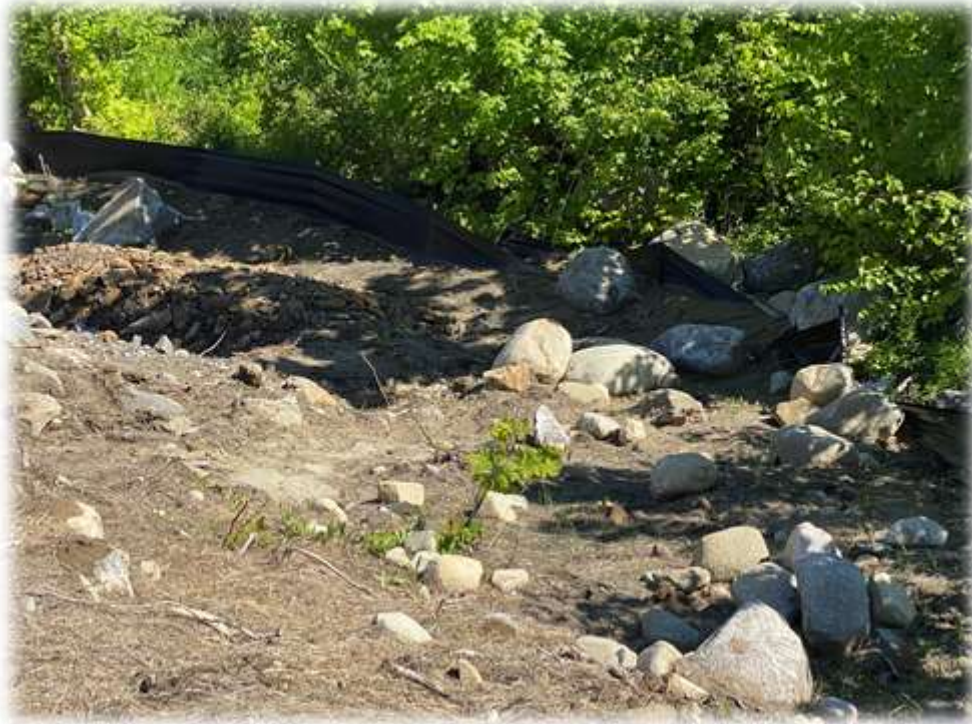
Photo #5: The silt fence along the toe of embankment along the access road curve near Tower 1 has captured significant sediment and needs to be cleaned. The sediment has topped the silt fence.
