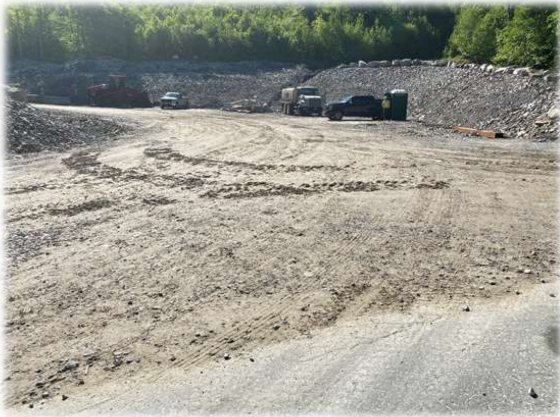
Photo #2: The stabilized construction entrance been removed in order to bring tower sections and blades into the project.
