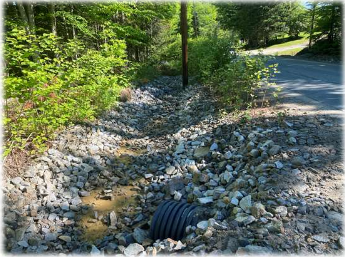
Photo #3: Water within the flow path along Horseshoe Valley Road is flowing as clear water. Some sediment lies along the top of stone.
