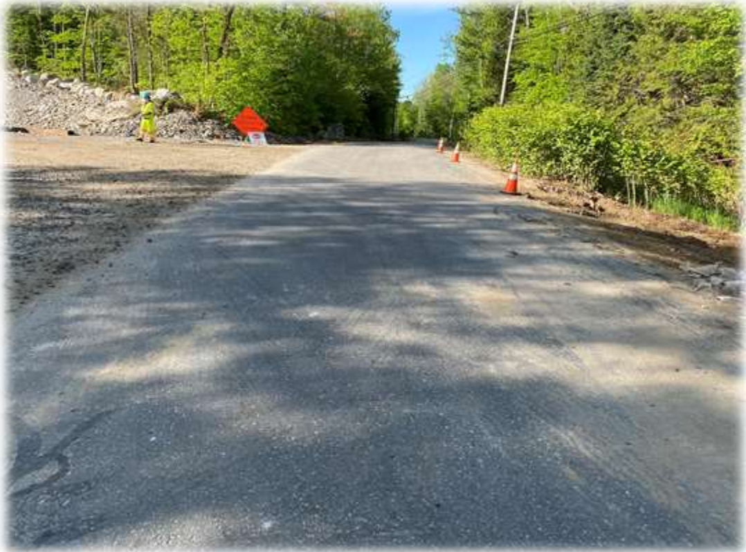
Photo #1: Horseshoe Valley Road is clear of soil debris from the project. The stabilized construction entrance still has some life left to the crushed rock entrance.
