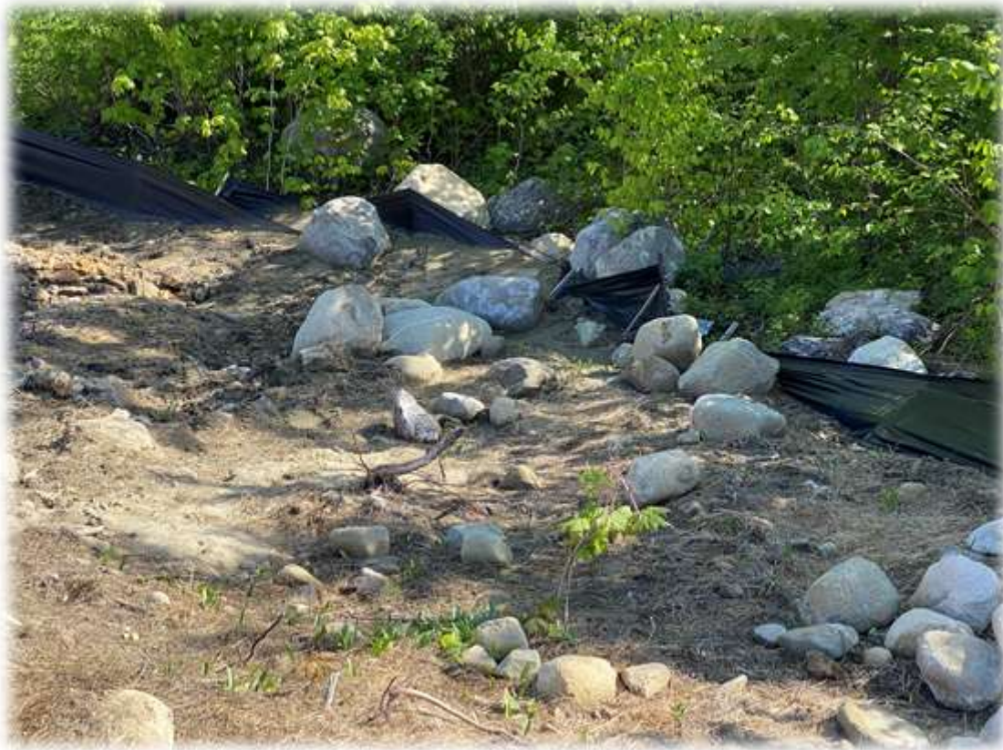
Photo #7: The silt fence has captured sediment (and large rocks) near the entrance to the corridor. It needs to be cleaned and silt fences reset to be functional again.
