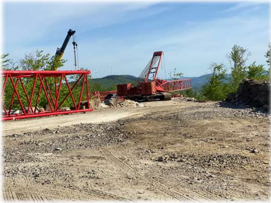
Photo #5: Action at Tower 1 includes assembling another big crane for tower work.
