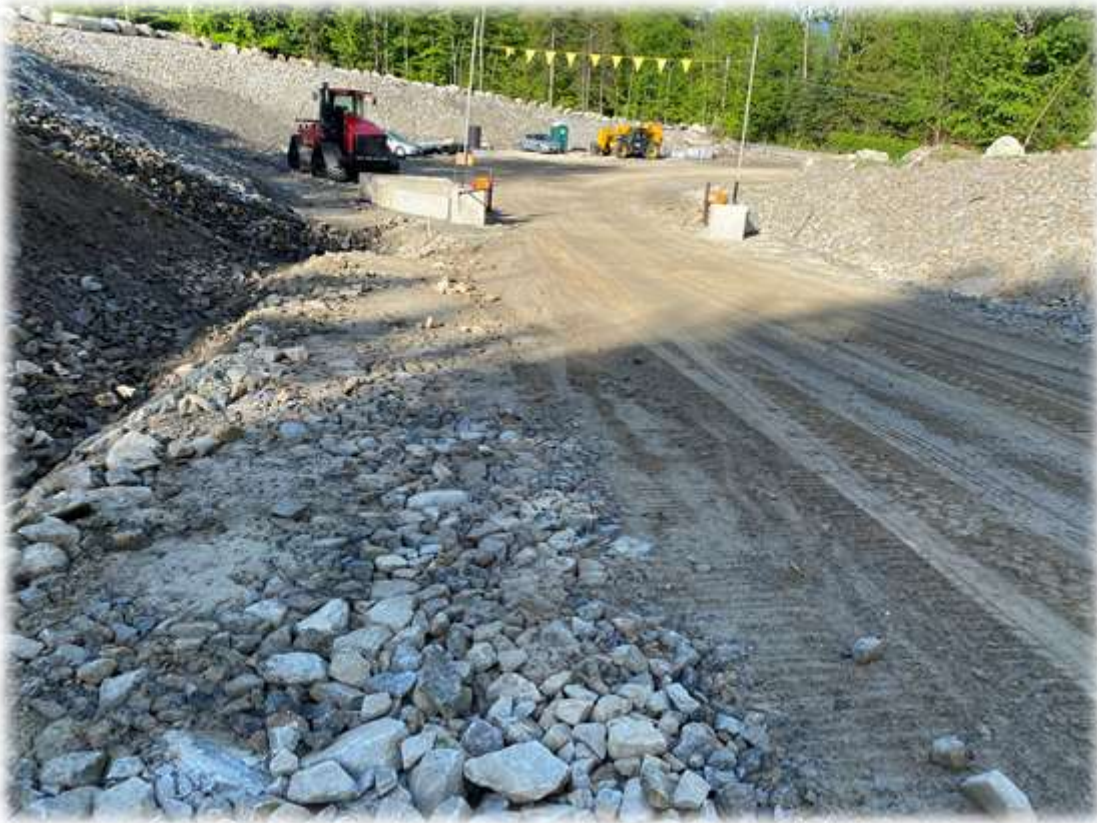
Photo #3: A groundwater breakout near the entrance gate along the access road has been repaired.
