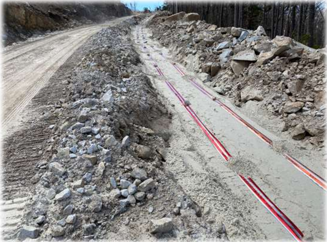
Photo #8: Marking tape for the buried electrical has been installed along the top of sand layer.
