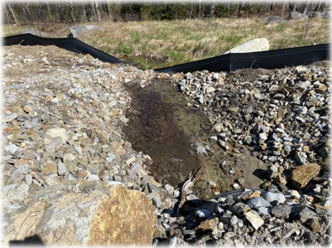
Photo #5: All of the culverts along the access road up to the top of the mountain are discharging clear water. Sargent is onsite and has cleared sediment/debris at the inlets and outlets of each pipe.
