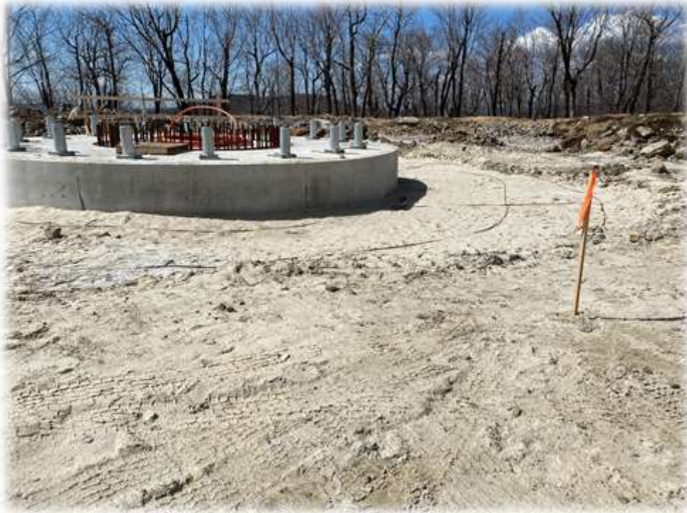
Photo #9: The Tower 4 base has been backfilled with sand and the grounding wire installed.
