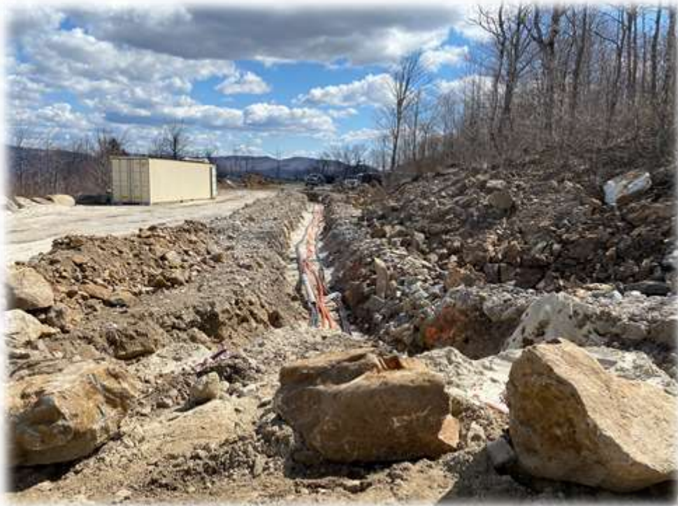
Photo #10: Conduit and direct bury electrical cables have been laid in the excavated trench and bedded in sand leading to Tower 2.
