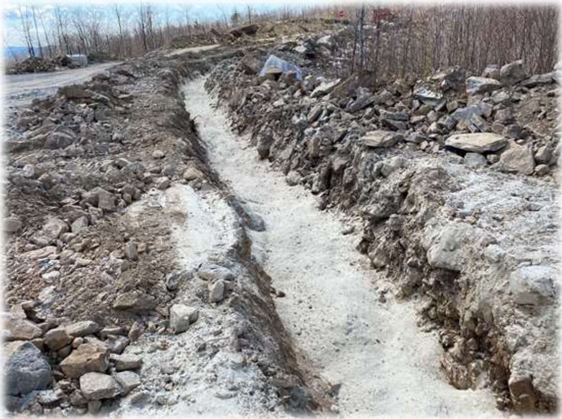
Photo #7: Trenching for the electrical cable conduit and backfill with sand has been completed to Tower 4. The trench backfill to final road grade is being performed this week.
