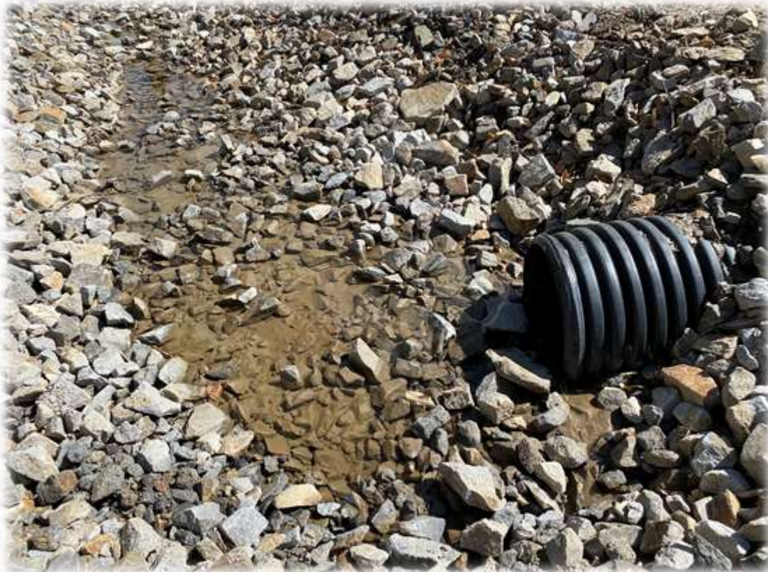
Photo #2: Water discharging from the Horseshoe Valley culvert near the entrance is crystal clear. There is some insignificant sediment within the plunge pool and culvert.
