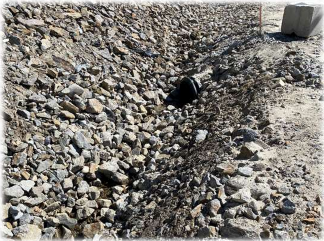
Photo #4: All of the culverts along the access road up to the top of the mountain are discharging clear water. Sargent is onsite and has cleared sediment/debris at the inlets and outlets of each pipe.
