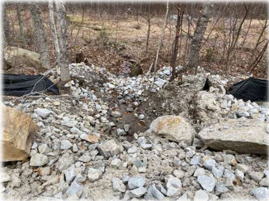
Photo #4: All of the culverts along the access road up to the top of the mountain are discharging clear water. Sargent is onsite and will check and clear sediment/debris at the inlets and outlets of each pipe as they work themselves up the mountain.
