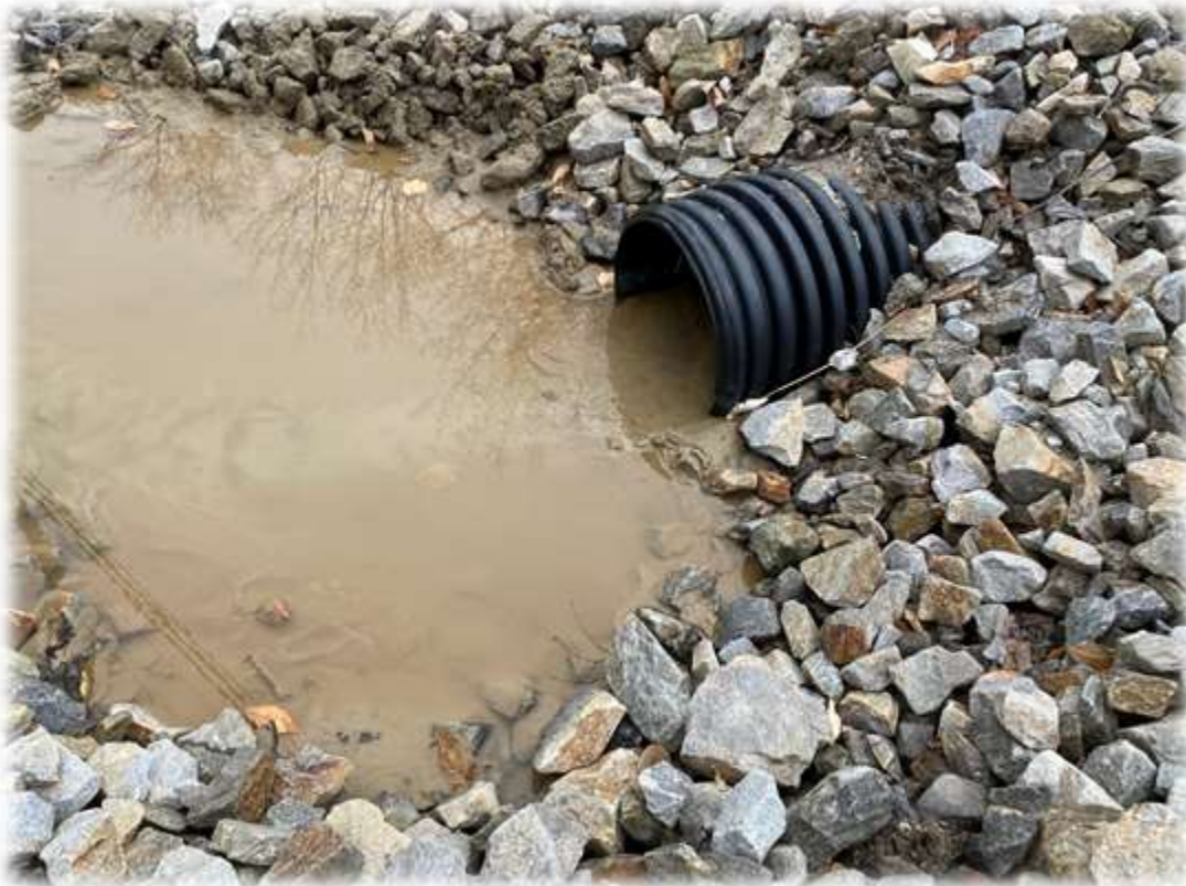
Photo #2: Water discharging from the Horseshoe Valley culvert near the entrance is crystal clear but there is significant sediment within the plunge pool and culvert. Sargent is onsite and is working to clear the winter sands from the upslope ditch and will clear (or reconstruct) this location last.
